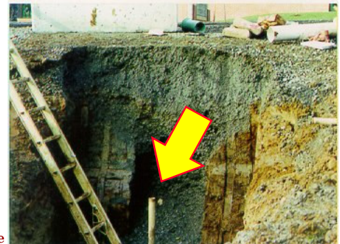
Watch for impalement hazards at base
