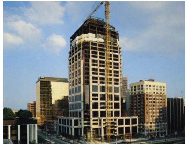
The 29-story First Indiana Plaza in downtown Indianapolis used 439,440 square feet of Vulcraft 3" composite deck.
