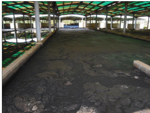
Figure 11. The reference bed, bed 0, at Lubigi sewage treatment plant five weeks after filling.
