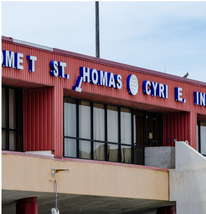
Damage from Hurricane Irma at the Cyril E. King Airport on St. Thomas
