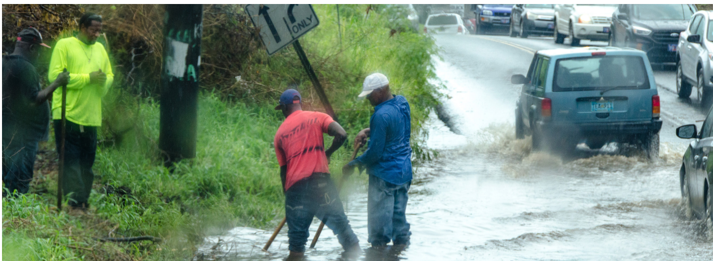
Workers clear debris from roadside drains during a rain storm to alleviate flooding on St. Thomas K.C. Wilsey/FEMA
