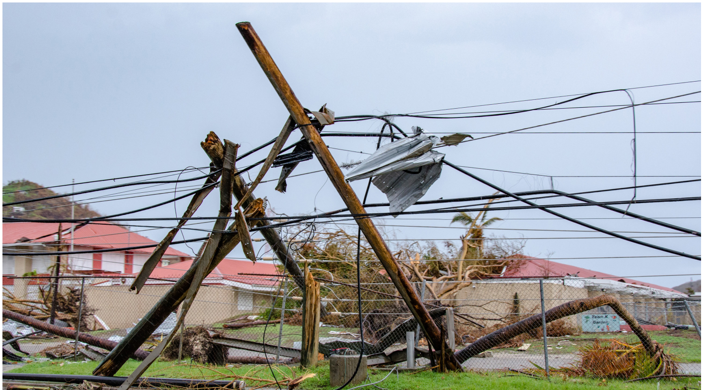
On St. Thomas, downed trees, snapped utility poles, and debris were evidence of the powerful winds from Hurricane Irma K.C. Wilsey/FEMA
