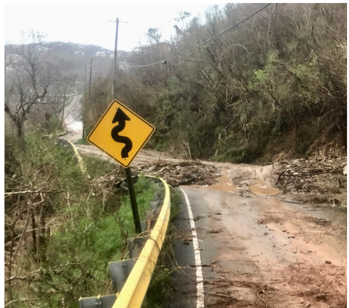
Damaged road on St. Thomas Kelsey Nowakowski
