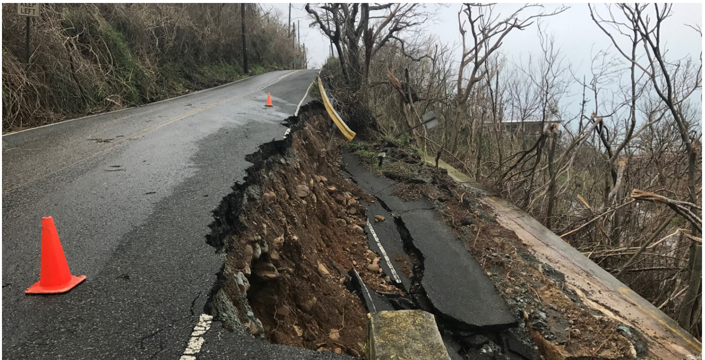
Hurricane damage to road in the USVI
