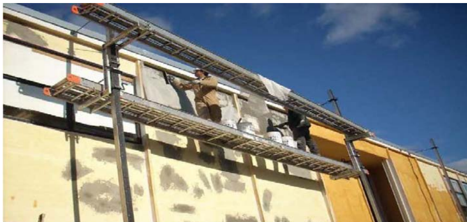
Figure 2: Base coat application: Touch-up on the first layer of stucco (left) and trimmed foam (right). The
