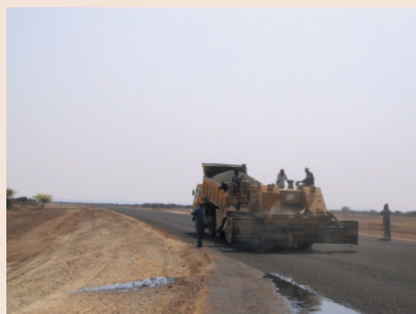
The surface sealing work may indicate that the project is close to completion.
