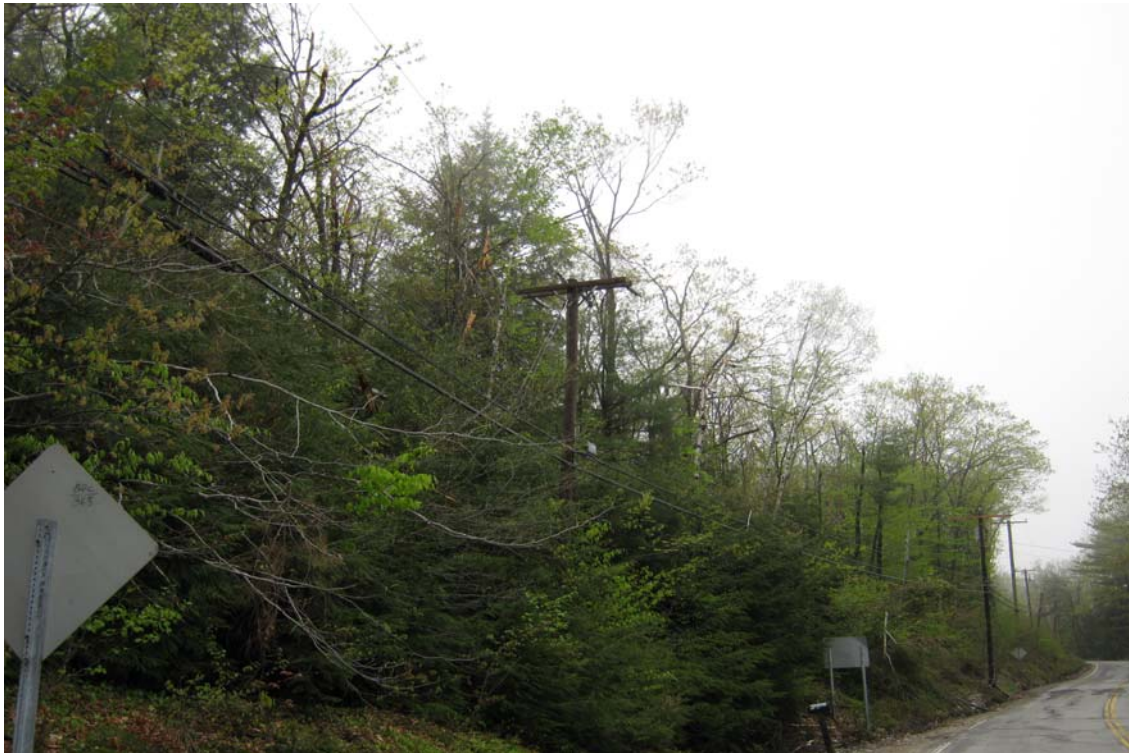
Figure IV-5 - Typical PSNH distribution circuit near Greenville, New Hampshire. (Photo by NEI - PSNH System)
