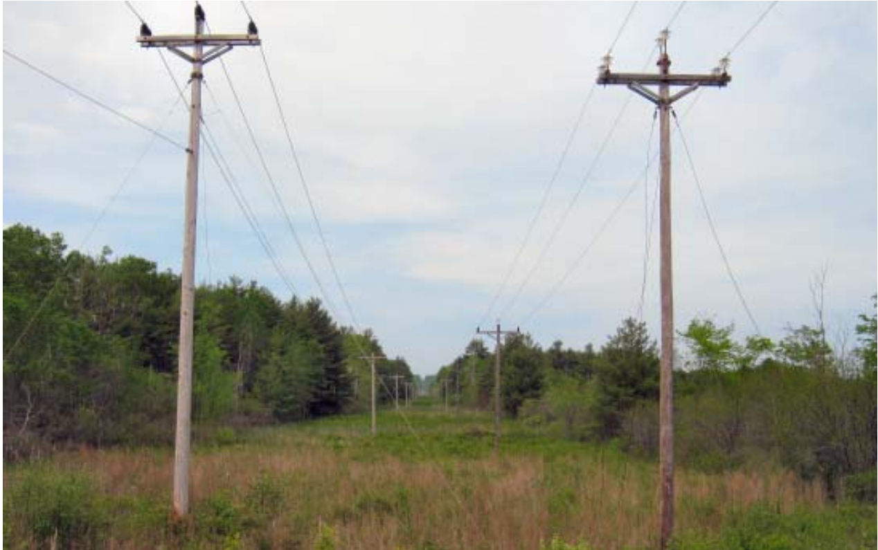
Figure IV-3 – Two 34.5kV sub-transmission lines located on the Unitil system. (Photo by NEI - Unitil System)
