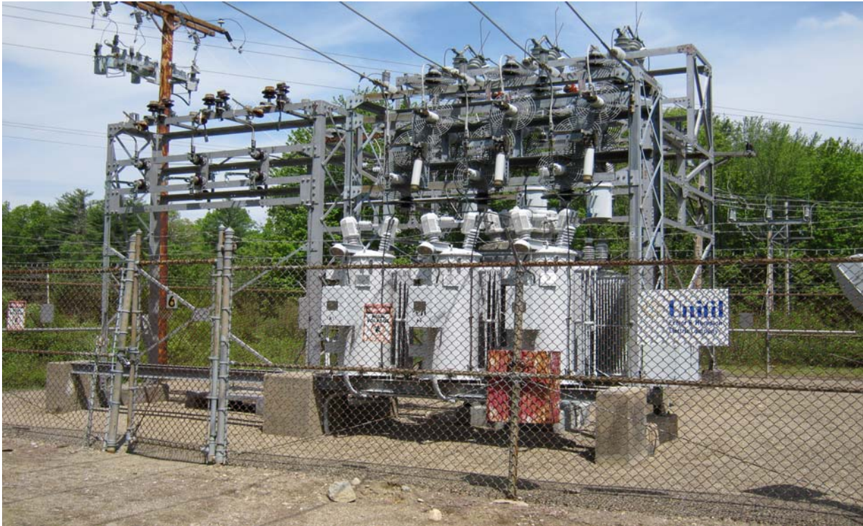
Figure IV-6 – 34.5kV to 13.8kV Unitil electric distribution substation located in East Kingston, New Hampshire. (Photo by NEI-Unitil System)
