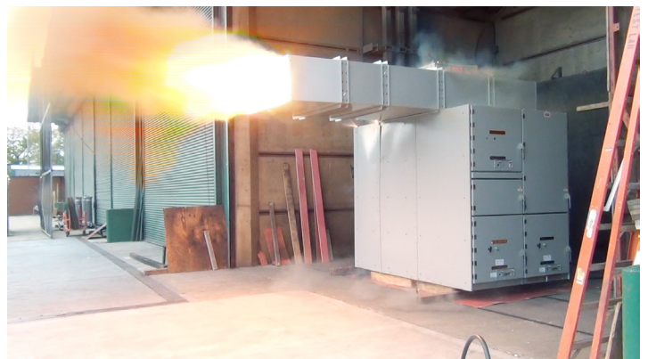
Plenum exhaust during arc event
