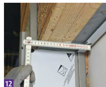
12 The head receiver strip is fitted and a measurement for the head flashing taken.
