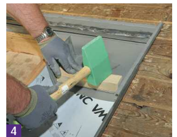
4 Complete double welt by gently hammering a wooden block onto the lower hem.
