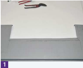
1 The window is traced onto back of the standing seam panel. A line 30mm back is drawn and then the zinc is cut out.
