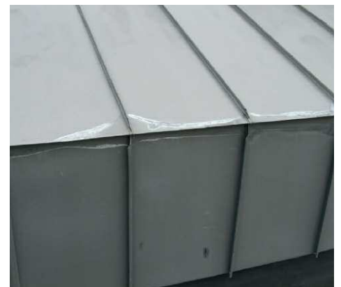
Staining resulting from partial removal of protective film.
