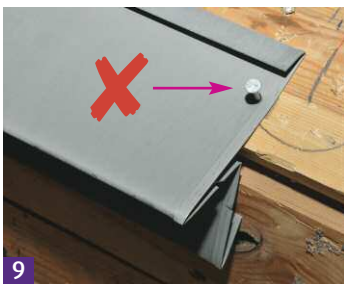
9 An eaves strip with a water check can also be used but must not be installed with a through fixing.
