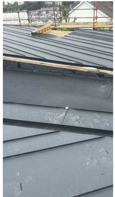
Boots should be cleaned prior to working on a zinc roof.
