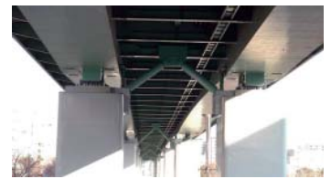
Nagoya Expressway: Elevated bridge falling-prevention device
