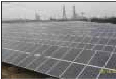
2010 8 MW Solar Power Plant
