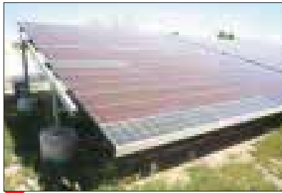
1985 150kW PV Inverter Running satisfactorily till date
