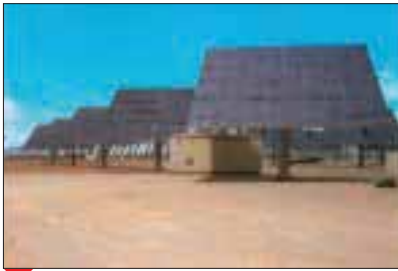
1985 1 MW Inverter Largest PV Inverter in the world
