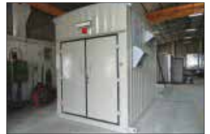
2011 20 MW Power Plant (2 Installations) 630 kW Inverters in the Package
