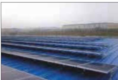
2015 20 MW Solar Power Plant
