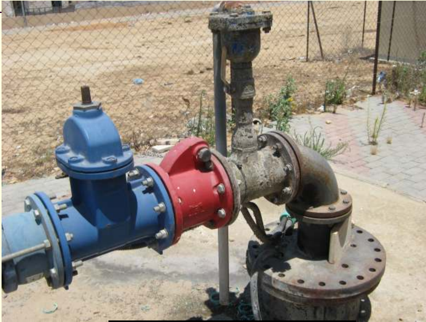
Submersible type motor installation
