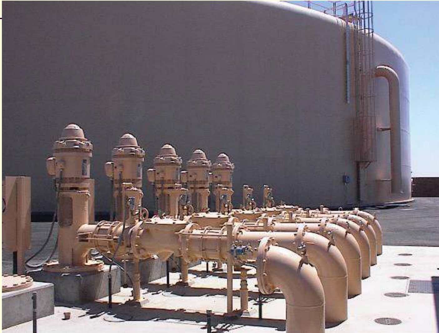
Distribution pumping station
