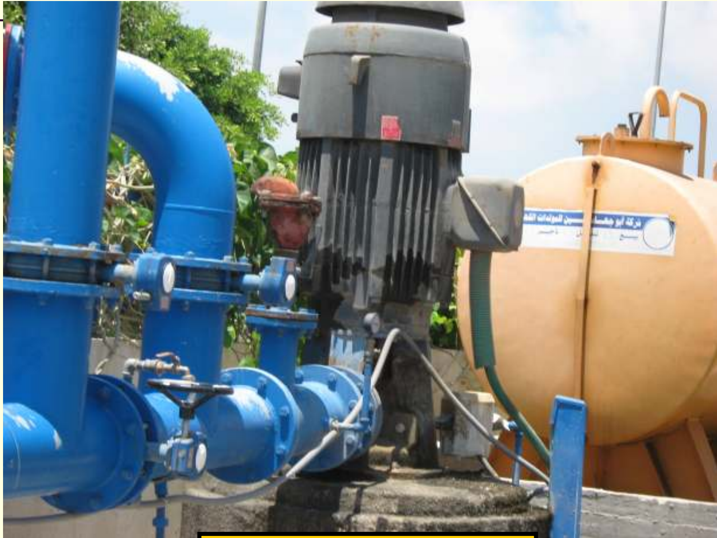
Vertical dry motor installation
