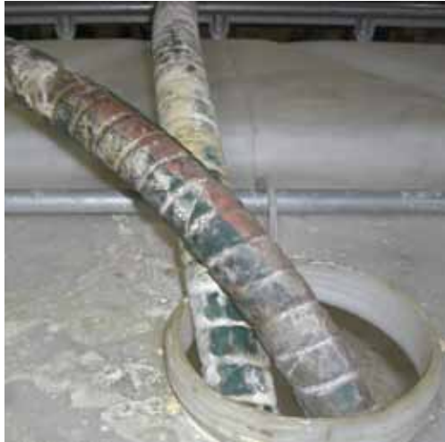
The outside of this bulk container and feeding lines, used to transfer an aqueous raw material slurry to the end product, must be kept clean. The residue on the outside acts as a nutrient source for micro-organisms. As is the case in this example, microbial growth could develop because of the high moisture level.
