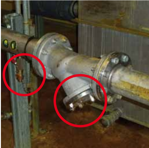
Bacterial growth on the outside of the piping. Decontamination of the outside of piping must form a part of the routine cleaning procedure. Please note that there are two areas where water can be trapped and result in standing water. These must be drained to prevent creating an optimal environment for microbial growth.
