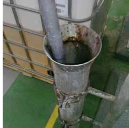
A filling lance for IBCs is stored after use in this wall mounted "bucket" without being drained and cleaned. Build-up of the residual liquid created ideal conditions for the growth of bacteria. Each time this lance was used, transfer of those bacteria to the next IBC took place.
