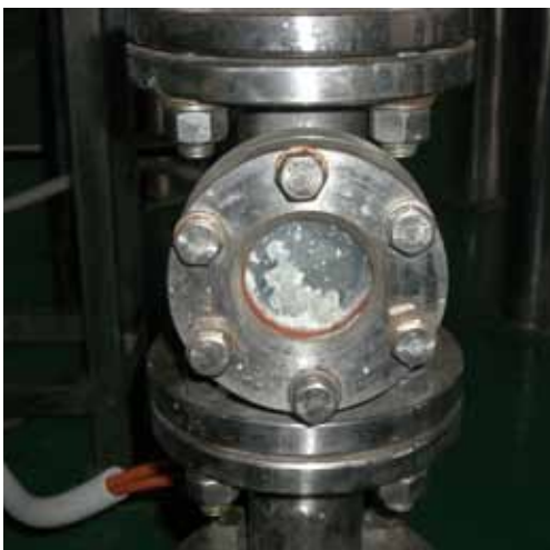
Sight glass in transfer line needs to be dismantled and cleaned after the finish of each production run.
