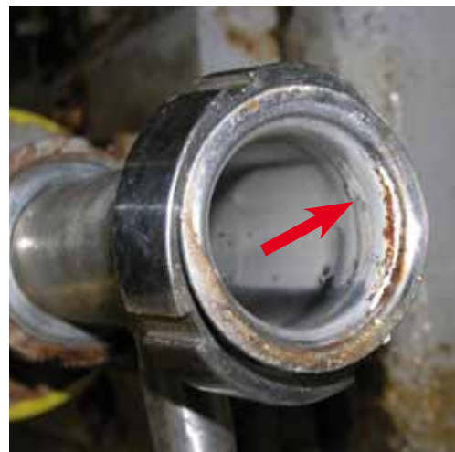
Poor welding of the coupling of a formulation line allowed for standing water in the pipe which is ideal for microbial growth.
