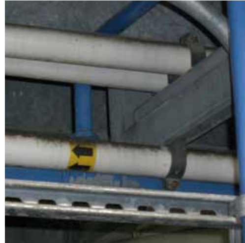
Another area where microbial growth could readily develop: on piping near the ceiling and thus partially out of sight. This must not be overlooked when carrying out a decontamination.
