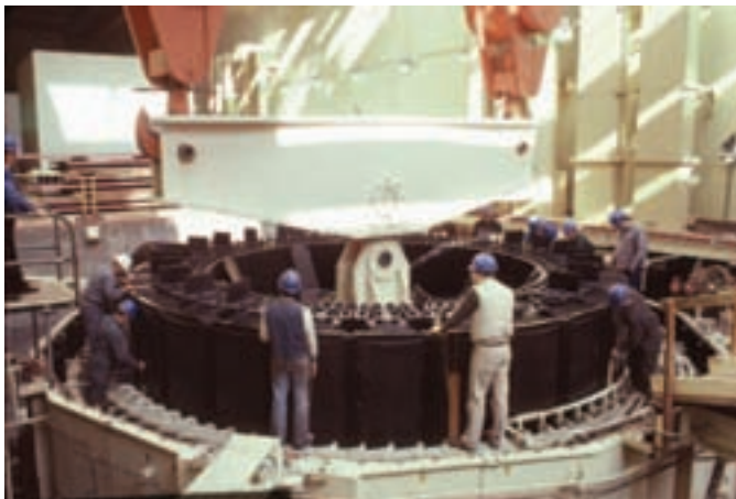
FIGURE 8.17 Turbine generator at Brown Mountain hydroelectric plant, shown during installation.
