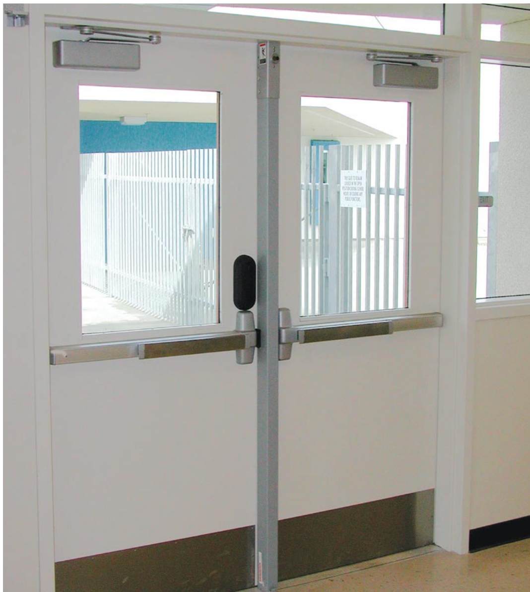
◀ Pair of doors includes Von Duprin 98 Series exit devices with Schlage WA993 lock on left, as well as LCN door closers and lockable Monarch removeable mullion to allow access for moving large objects and equipment.
