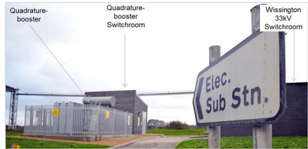
Figure 4: Picture of the Wissington substation site showing location of installed Quadrature-booster
