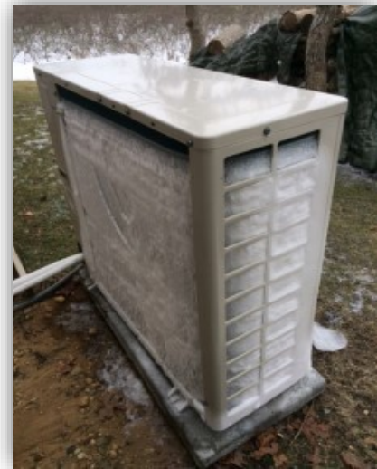
Pictured Above: A frozen outdoor condensing unit. This can be caused by air flow blockage or lack of refrigerant.
