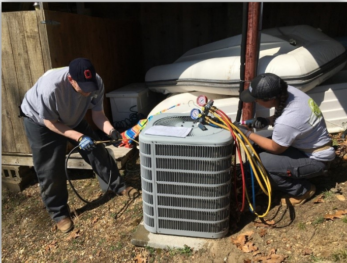
Pictured Above: Two of our professional HVAC technicians checking pressure on the outdoor condenser to make sure the system is operating correctly .
