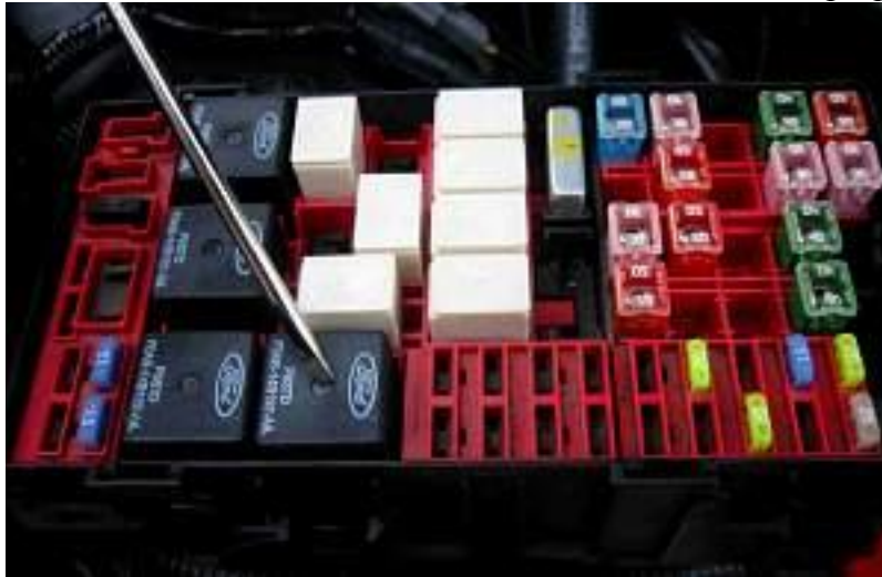
Picture showing relay # 301
