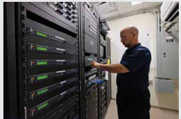
VMware server virtualization enables North Las Vegas to improve city services and save millions of dollars.
