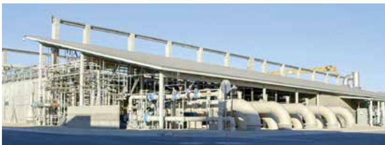
The city's fully-virtualized, IoT-based, state-of-the-art water treatment plant.
