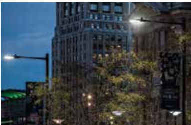
City Streetlights with Flashnet Controller on Top
