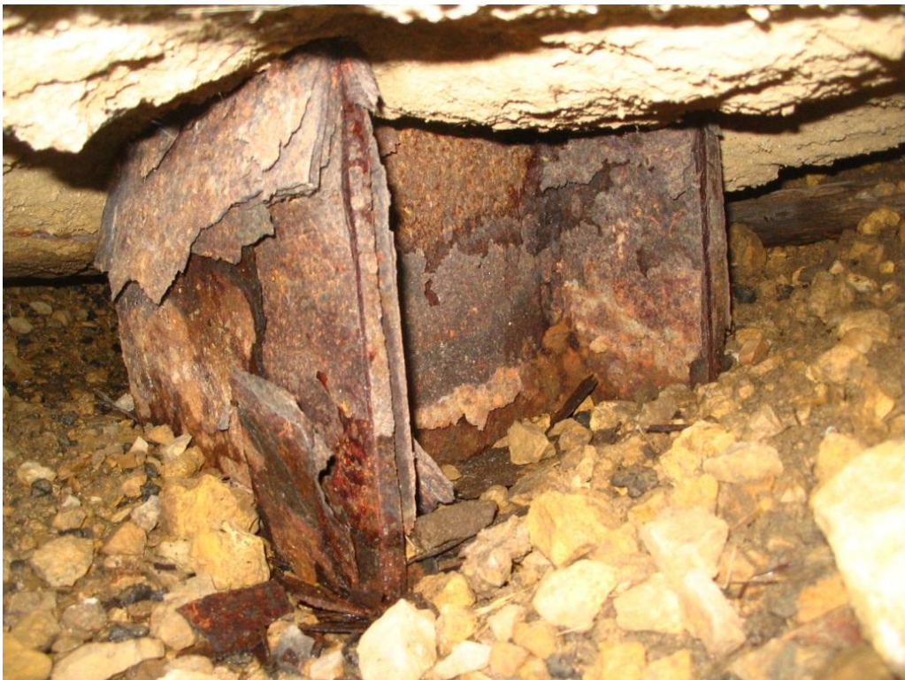
Figure 4. Laminar corrosion at bridge pile
