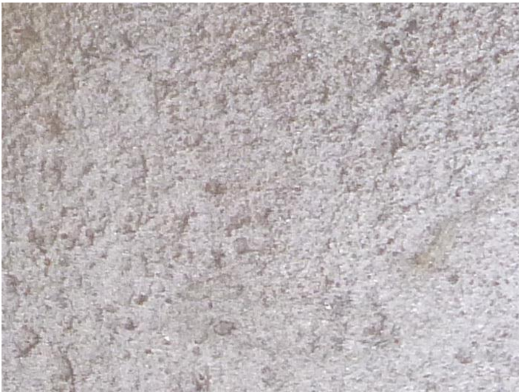
Figure 30. Typical abrasive blast cleaned surface at relatively difficult to reach area of pile
