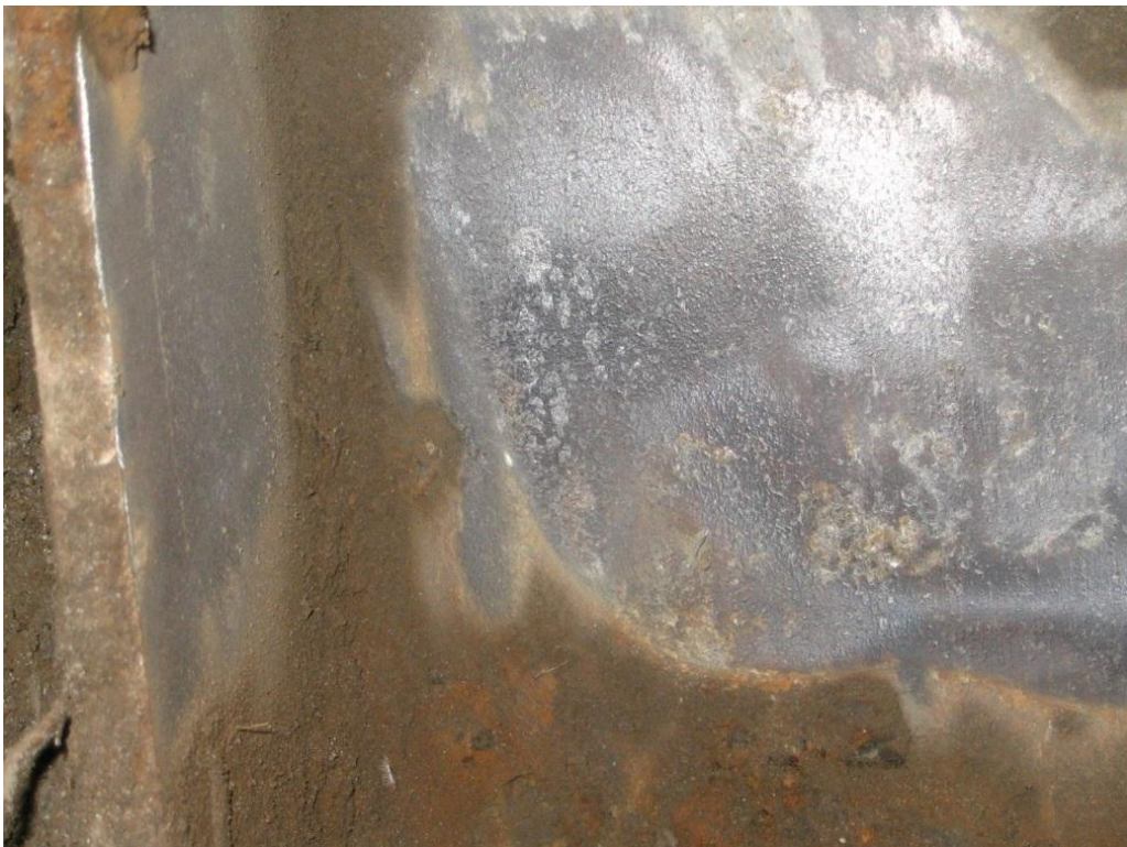
Figure 6. Covered pile after excavation with little corrosion
