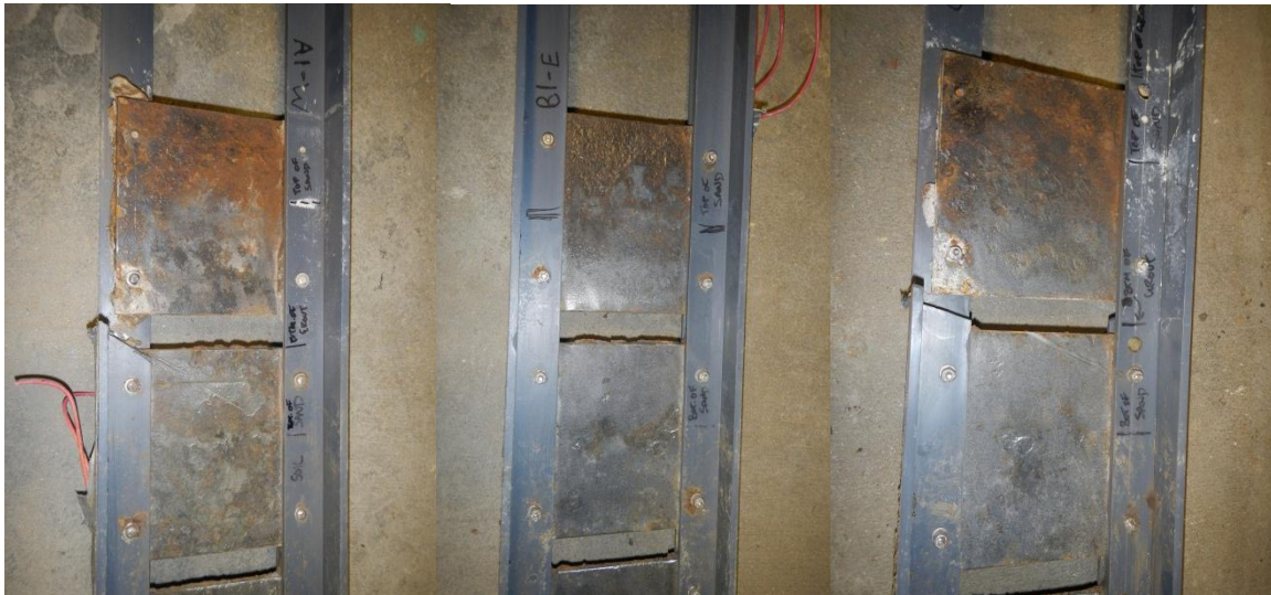
Figure 61. Close-up view of top plates of each pile after cleaning with wire brush
