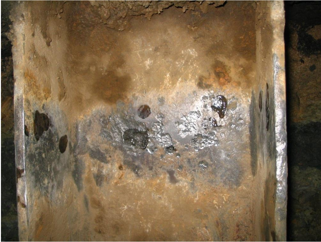
Figure 5. Pitting in bridge pile
