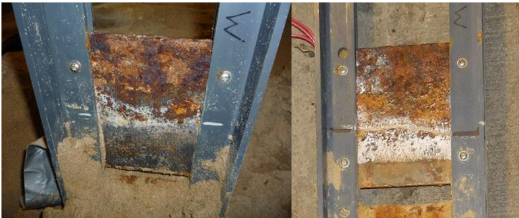
Figure 64. Plate 1 of Pile B before and after mortar blocks on other piles (top of sand is white line). Note: no mortar was installed on Pile B.
