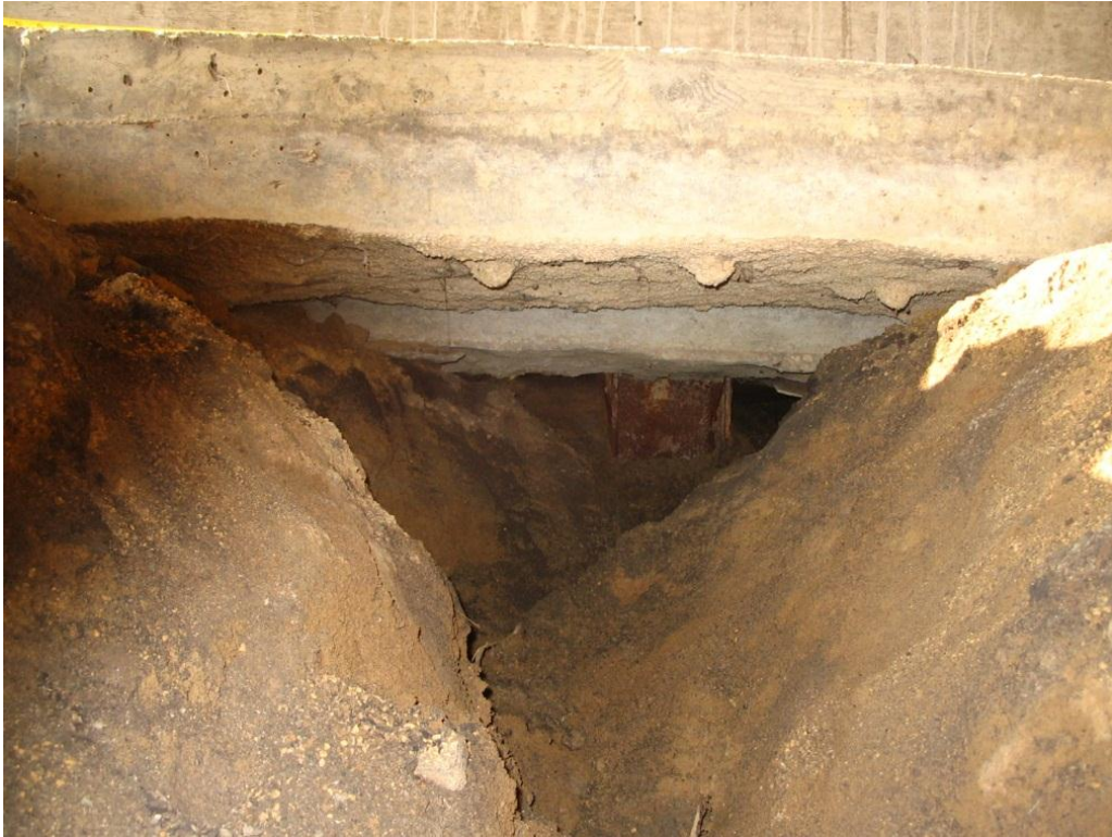
Figure 1. Erosion and exposed pile at bridge abutment
