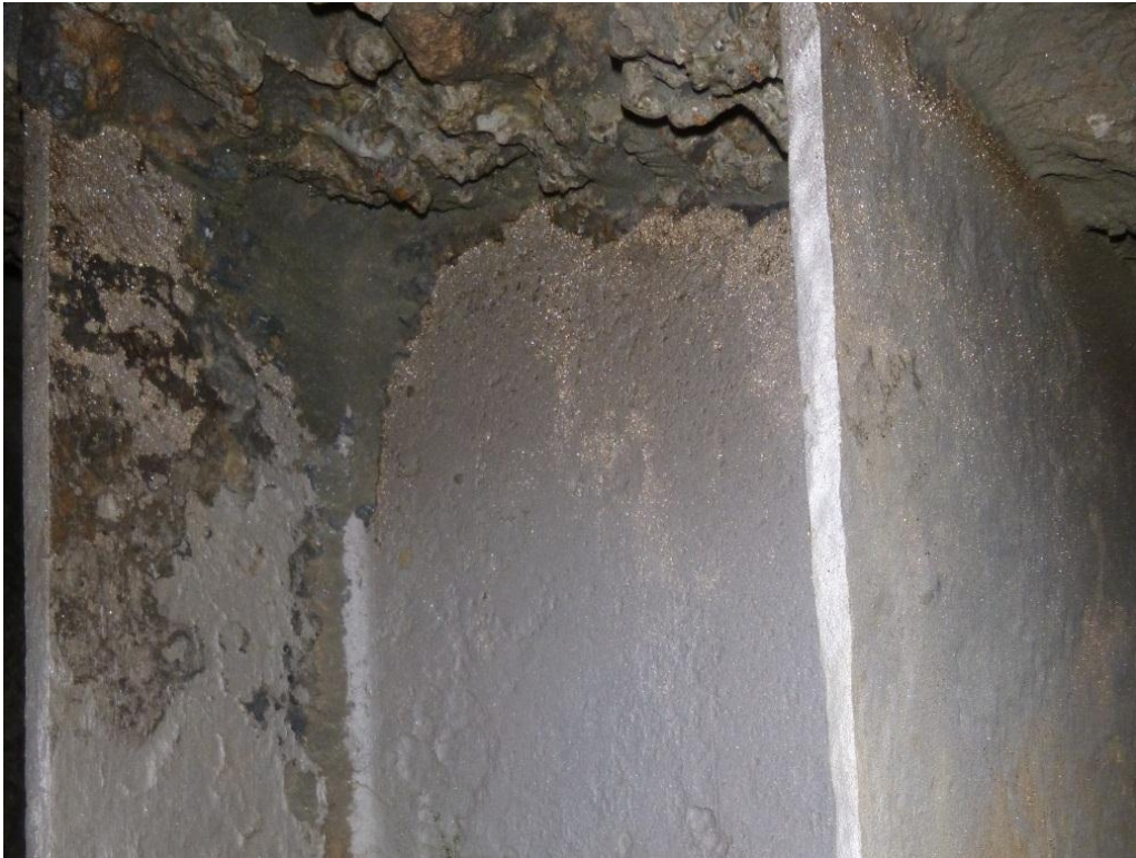
Figure 29. Example of difficult-to-reach location on pile requiring additional cleaning effort. Note remnants of clay soil in corner of web, flange, and footing.
