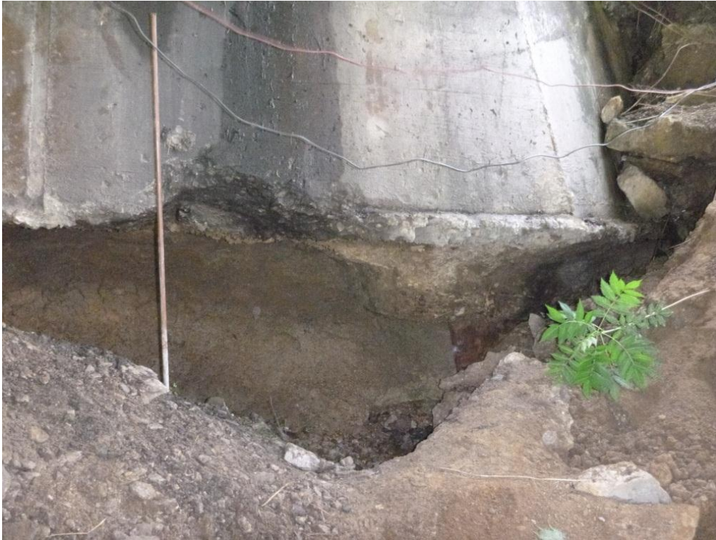
Figure 25. Erosion at north end of west abutment of Bridge No. 9081.5S034
