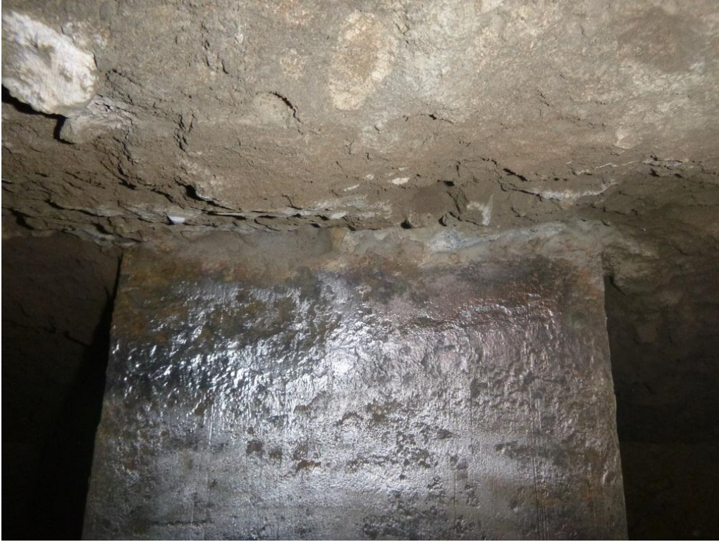
Figure 33. Pile/abutment interface inaccessible for surface preparation with MBX Bristle Blaster
