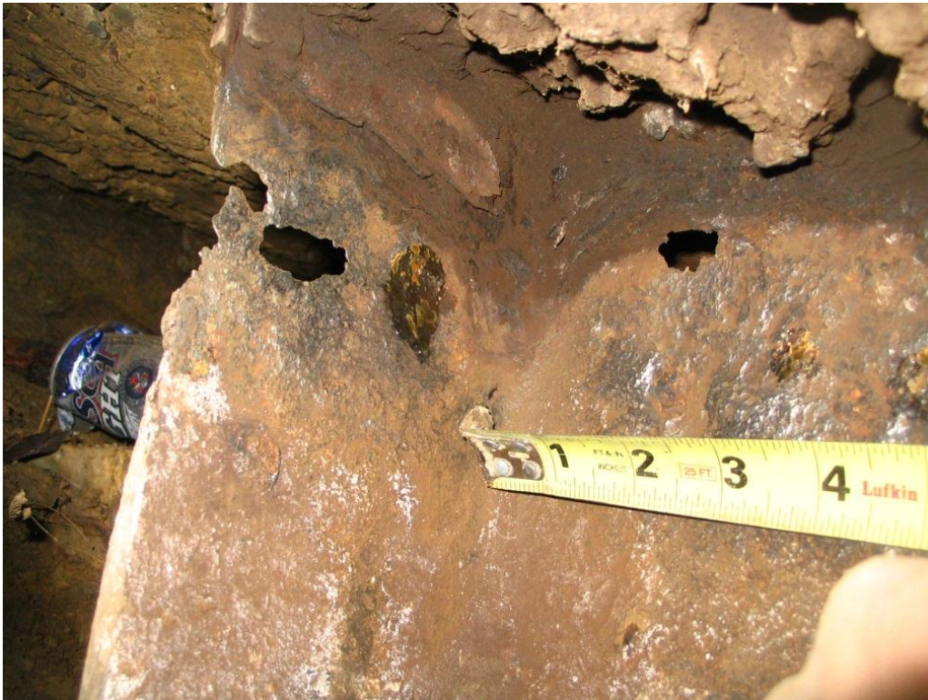
Figure 7. Perforations in flange and web of exposed pile
