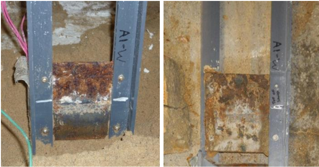
Figure 63. Plate 1 of Pile A before and after mortar block (top of sand is white line).
