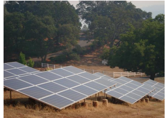
18Kw owned & installed solar array
