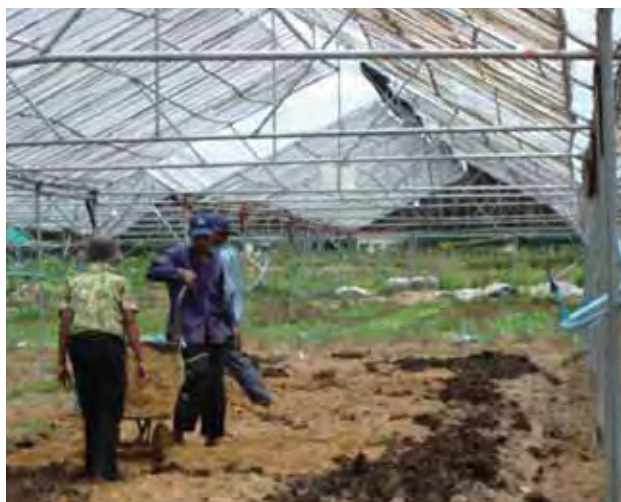
Soil and peat being placed into the greenhouses to raise and even the beds
