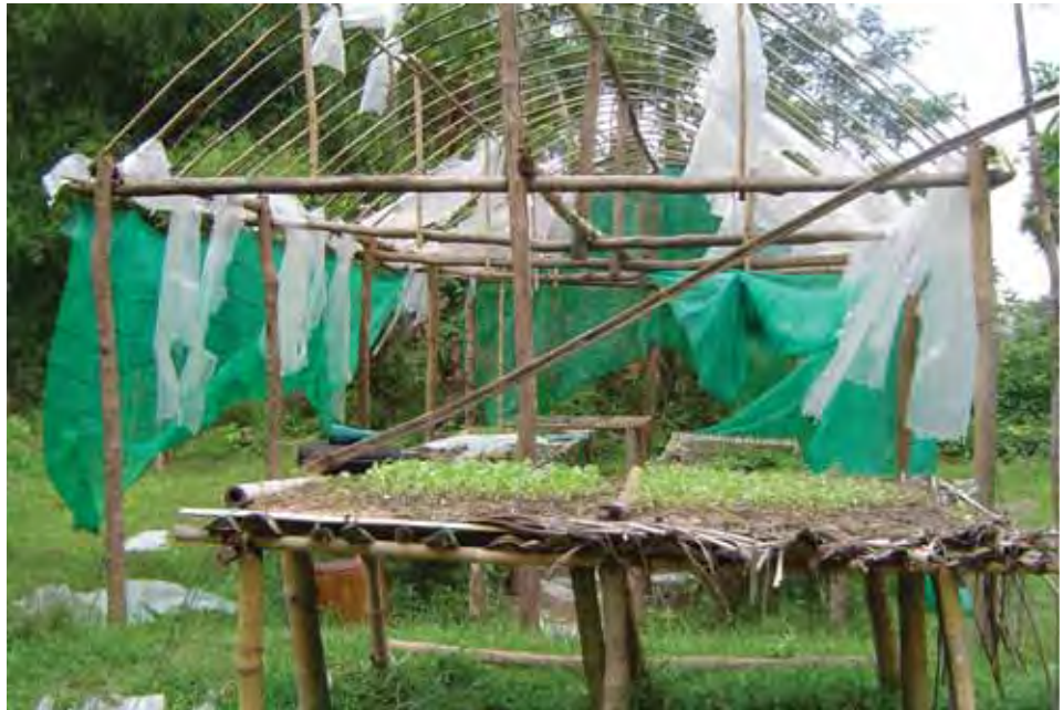
Greenhouse damaged by heavy rains. Village farmers need to put money aside to maintain shared assets.
