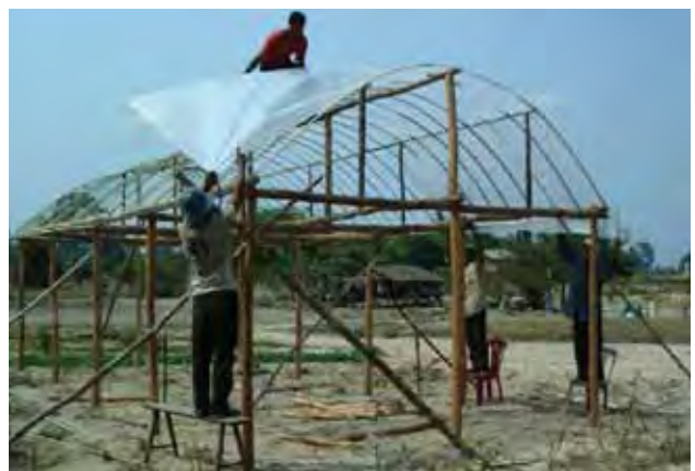
ILO-sponsored village nursery being constructed by the farmers of Plung Village, Angkor Thom District
