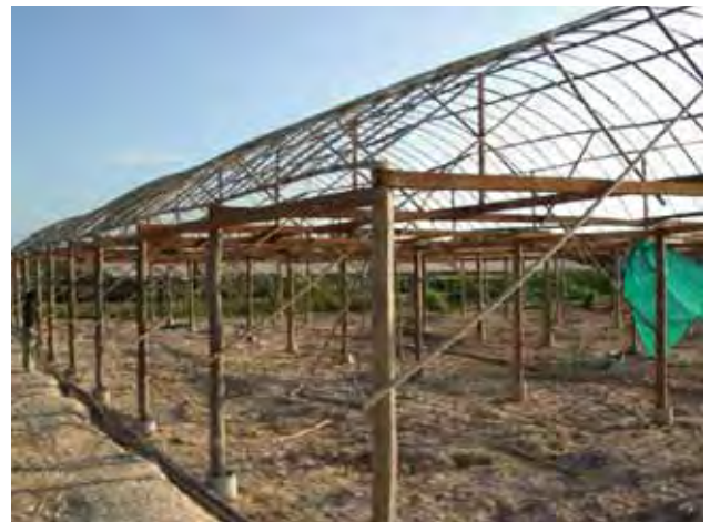
Construction of the new greenhouse complex with all locally-produced materials (timber and bamboo) in contrast to previously used steel bars
