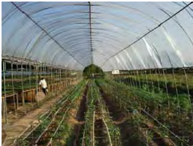
The new German funded greenhouse being constructed beside the nursery (this is a demountable steel design secured by spring steel clips)
