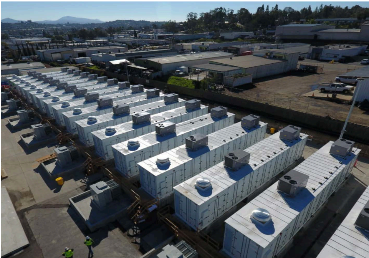
Figure 6 AES 30 MW (120 MWh) Li-Ion ESS Installation in San Diego, CA [19]
