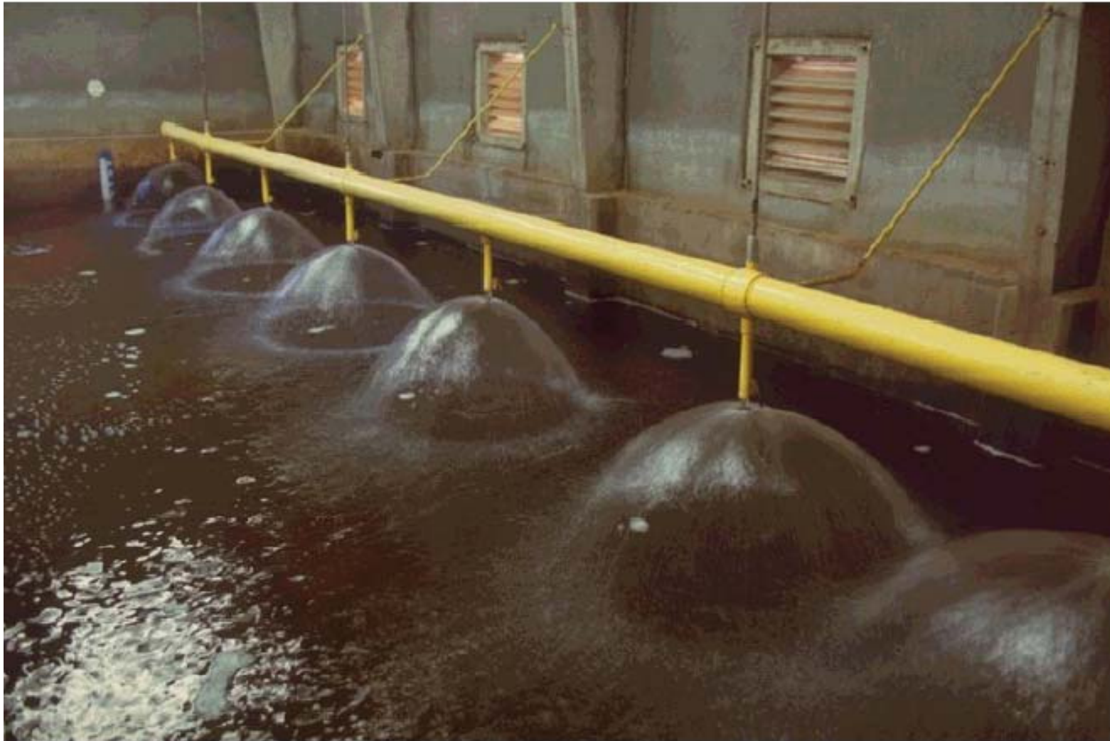
Spray Aerators: Nozzles
