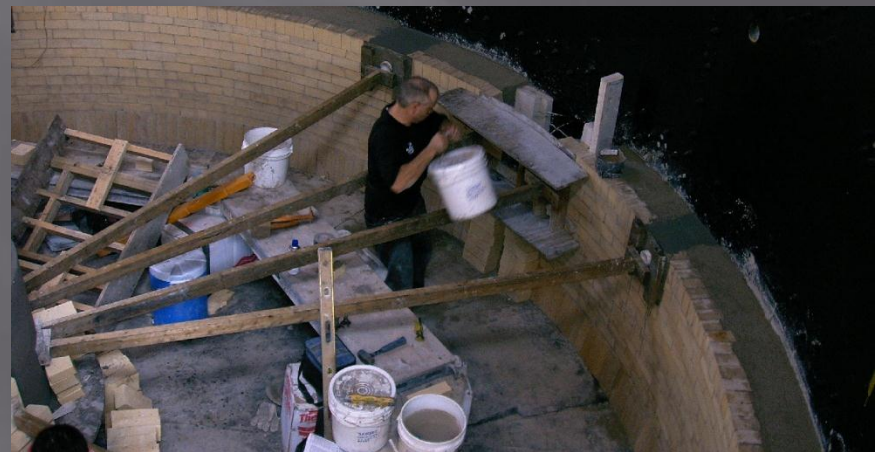
A crew installing a new furnace wall lining and hearth. In this photo they are pouring a refractory burner tile.
