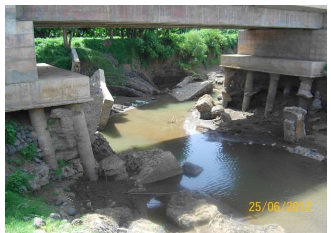
Figure.2.2. Scour at Sile River Bridge
