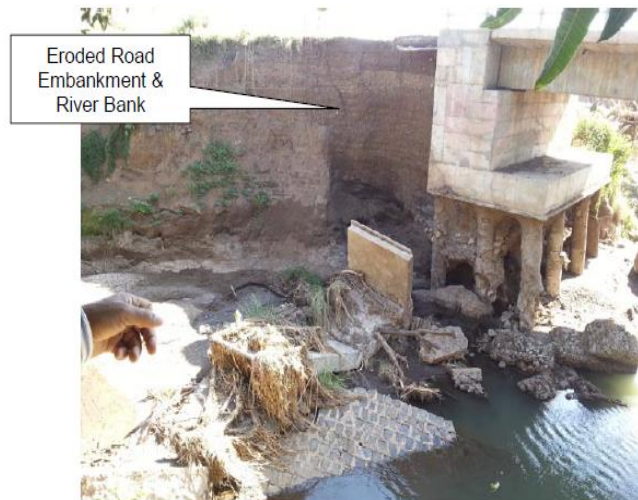
Figure 2.4. Damage on the left bank by the October 2012 flooding.
