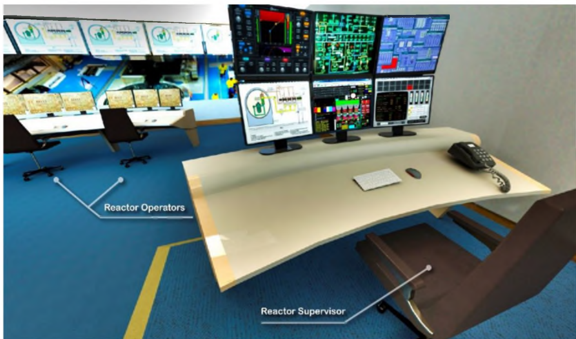
Figure 2: The main control room
