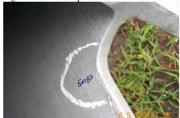
Figure 9. Cope Crack in Beam
