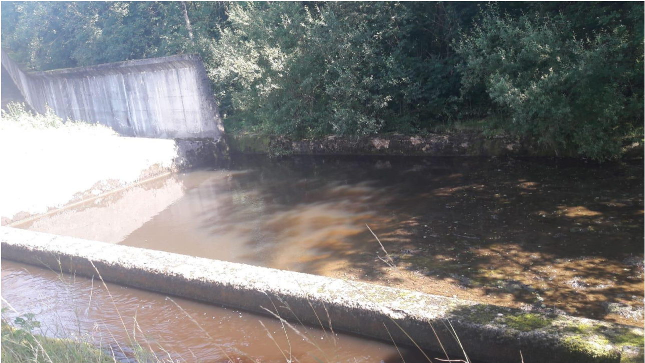
Figure 6.2: Photo looking upstream showing outfall of spillway, adjacent to compensation channel (foreground)
