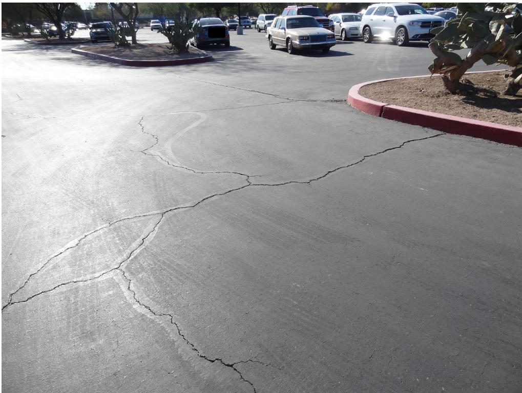
Grant Sawyer Office Site - Site #9835 Description: Asphalt Crack Fill & Seal Needed
