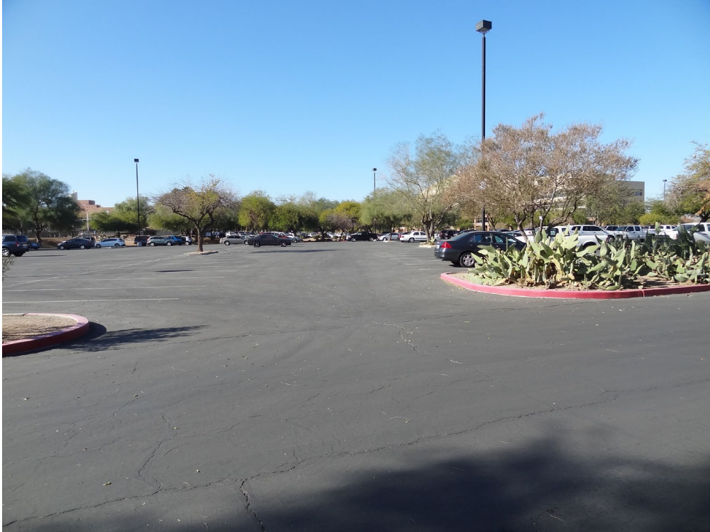
Grant Sawyer Office Site - Site #9835 Description: Site Lighting Upgrade Recommended.
