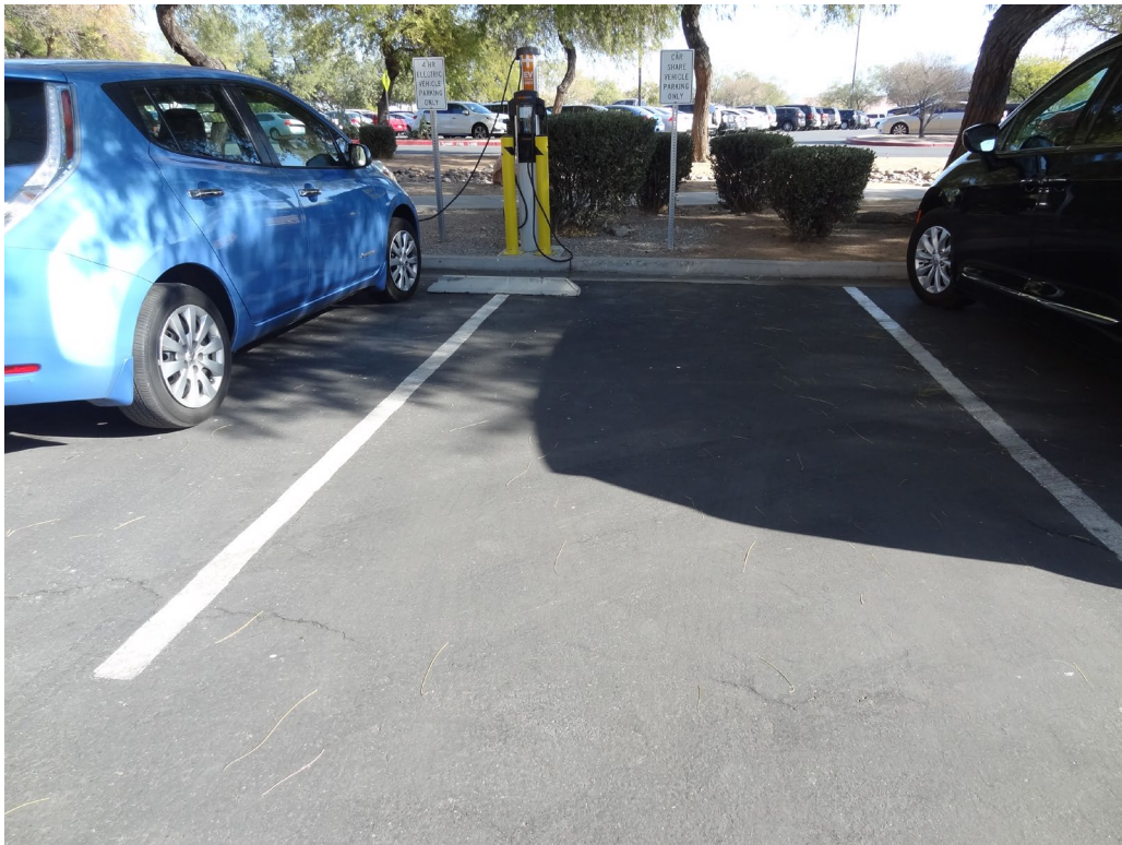
Grant Sawyer Office Site - Site #9835 Description: View of Electric Vehicle Charging Station.
