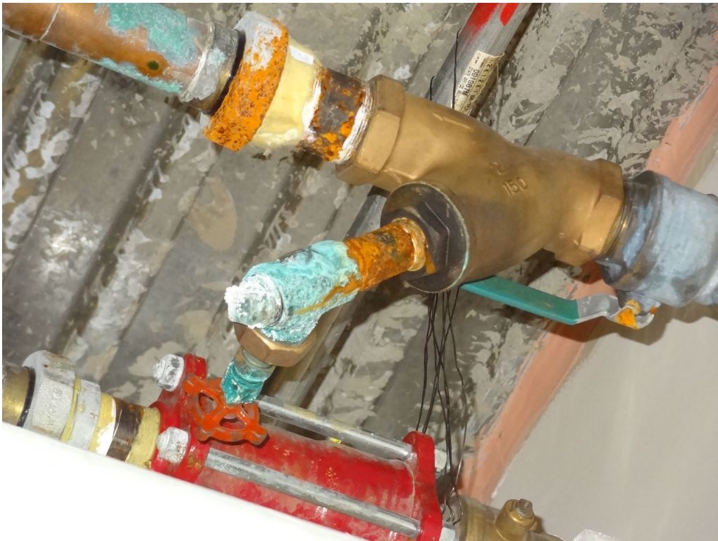
Grant Sawyer State Office - Building #1680 Description: Mechanical Piping Replacement Needed.
