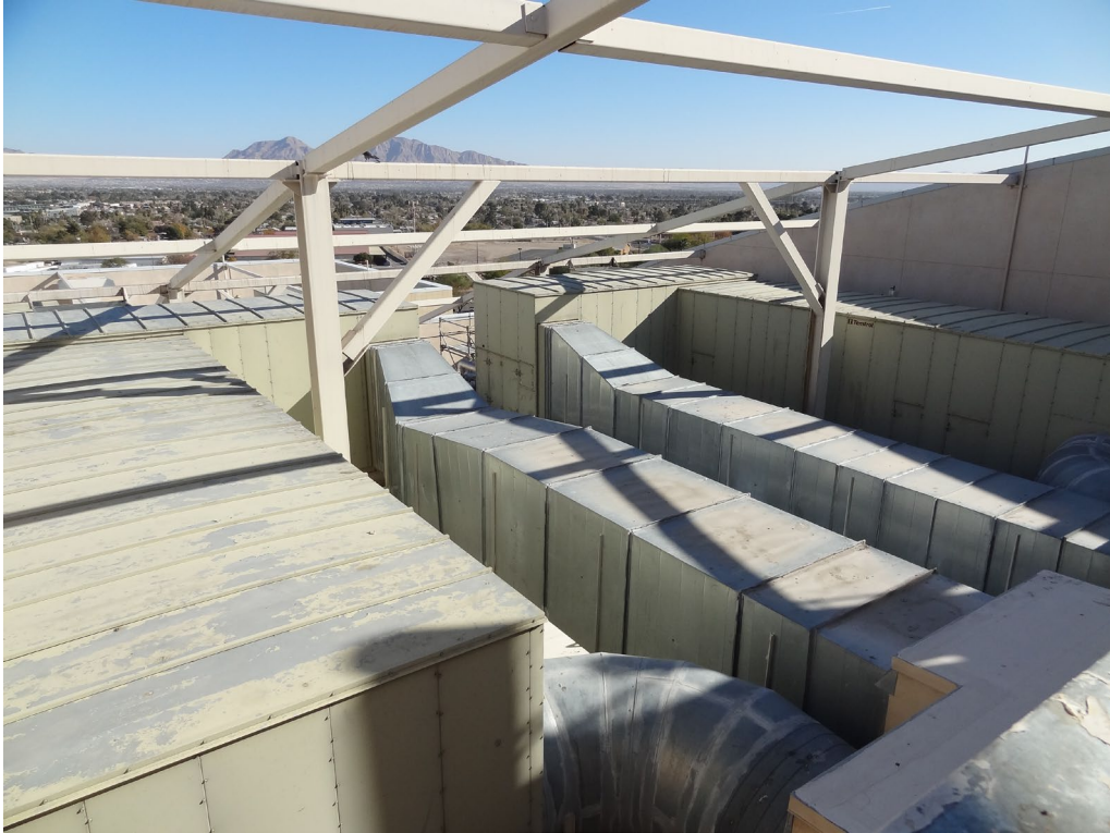
Grant Sawyer State Office - Building #1680 Description: Air Handling Units & Exterior Ductwork Needing Replacement.
