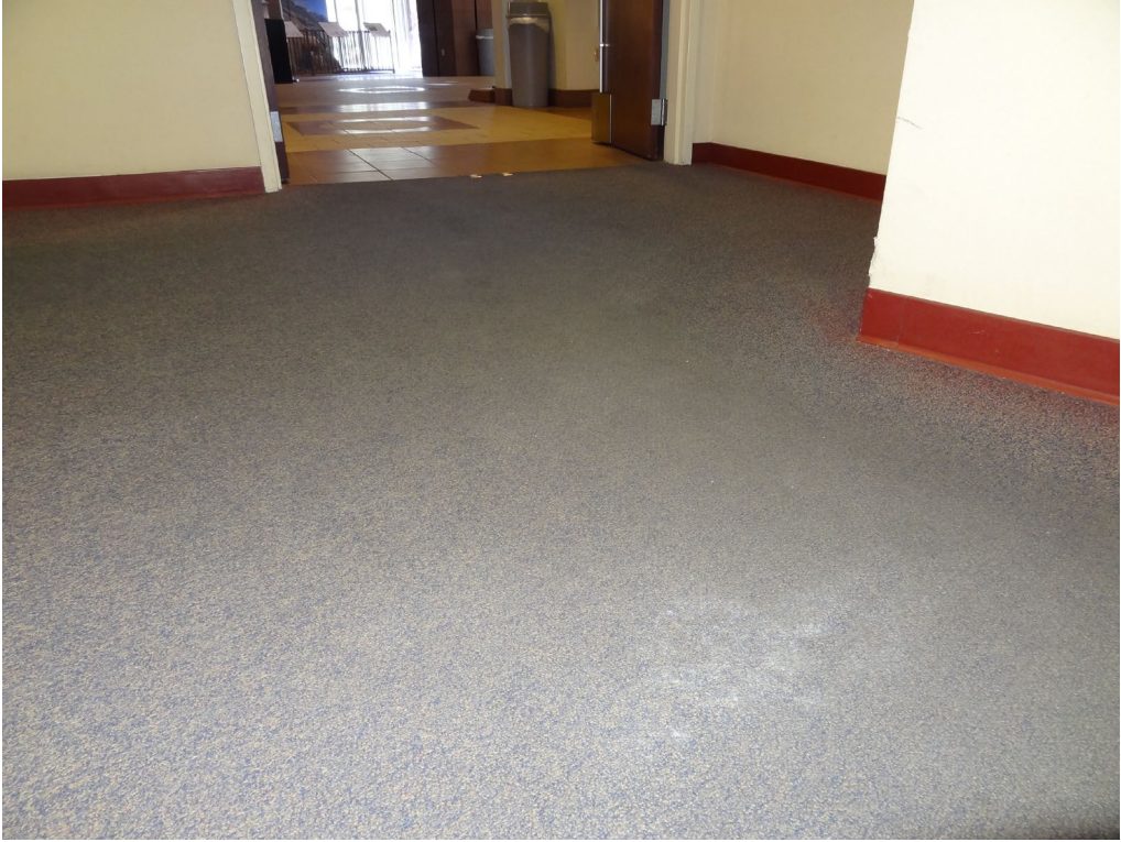
Grant Sawyer State Office - Building #1680 Description: Flooring Replacement Needed.
