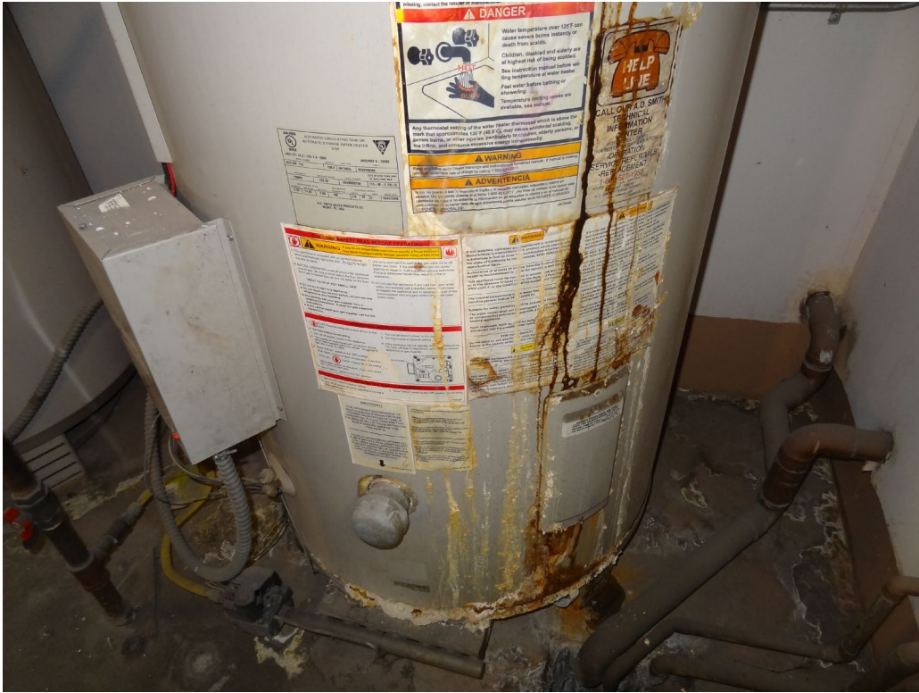
Grant Sawyer State Office - Building #1680 Description: Water Heater Replacement Needed.
