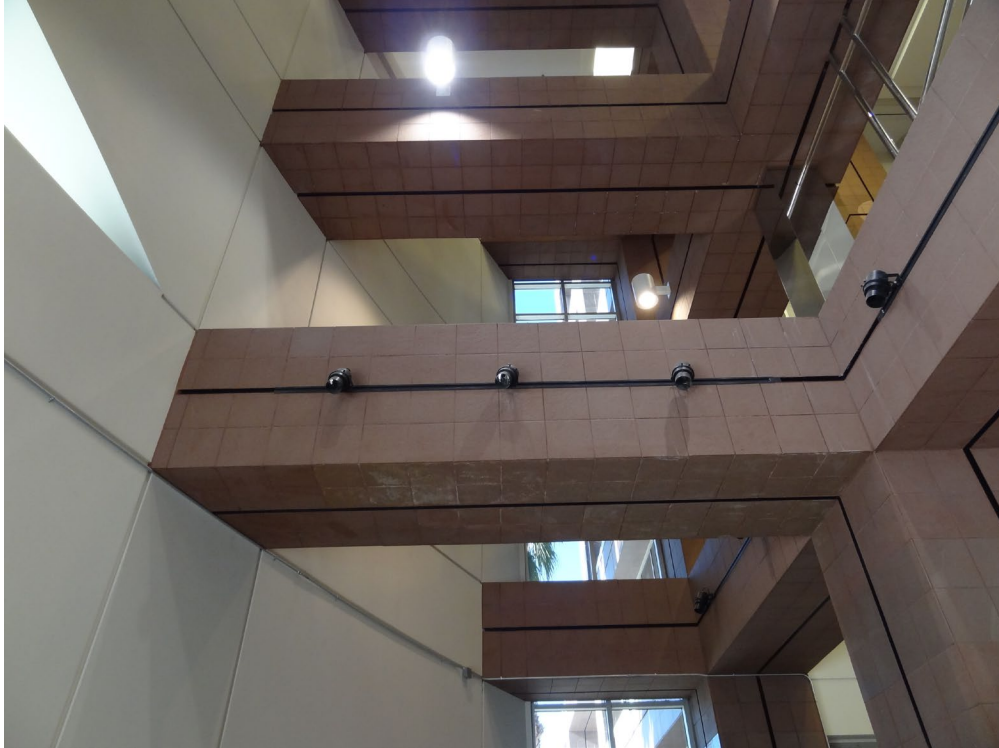
Grant Sawyer State Office - Building #1680 Description: View of Interior and Interior Finish Issues.
