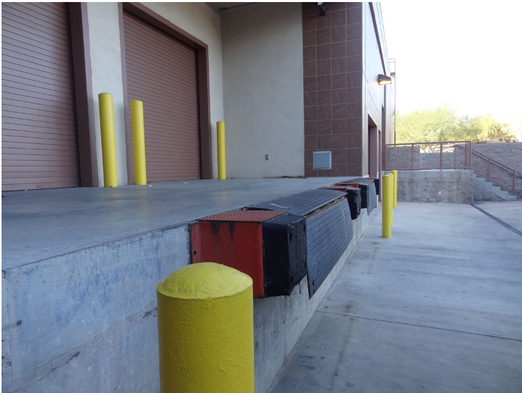
Grant Sawyer State Office - Building #1680 Description: Loading Dock Lacking Parcel Delivery Size Ramp.
