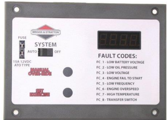
Panel inside of generator
