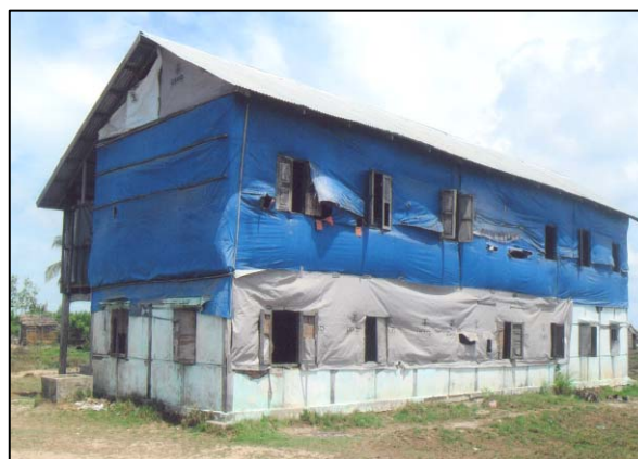
A temporary school in Ayeyarwaddy Delta before repair works after Nargis
