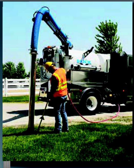
Standard wireless boom and air compressor
