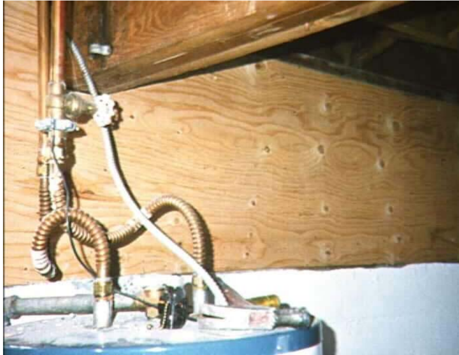
Figure 11 Refer to Drawing Detail 2d to determine how to cut-out a section of the structural panel to accommodate piping, etc. (Photo from Ben Emam)
