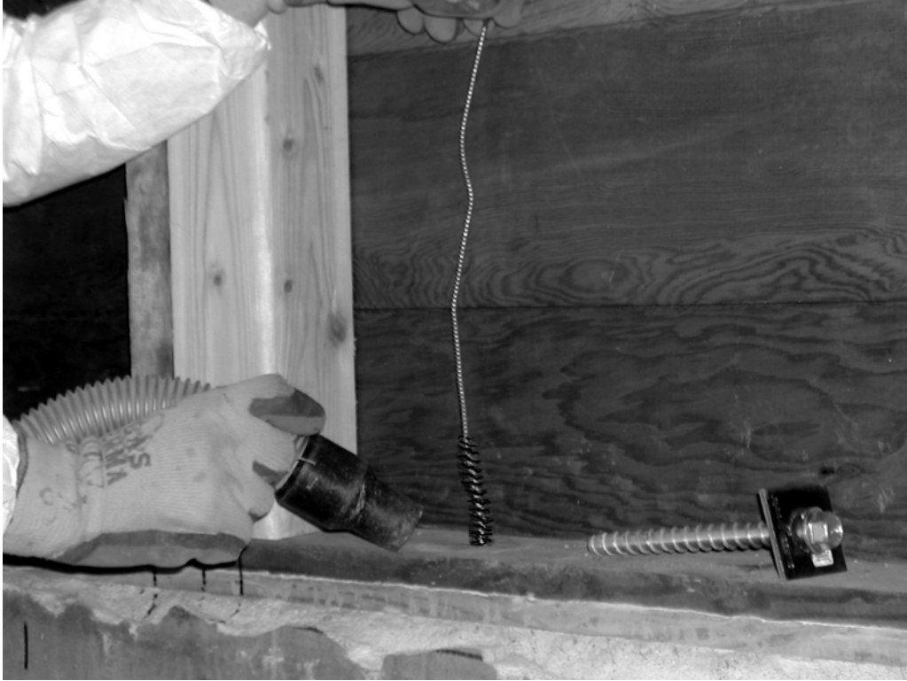
Figure 6 Mechanical anchor bolt for connecting the sill plate to the foundation wall. Note that square plate washers are required. In this photo, worker is cleaning out drilled holes using a brush and a vacuum. Also note the importance of protective safety equipment being used in these photos. (Photo from Tom Hall)
