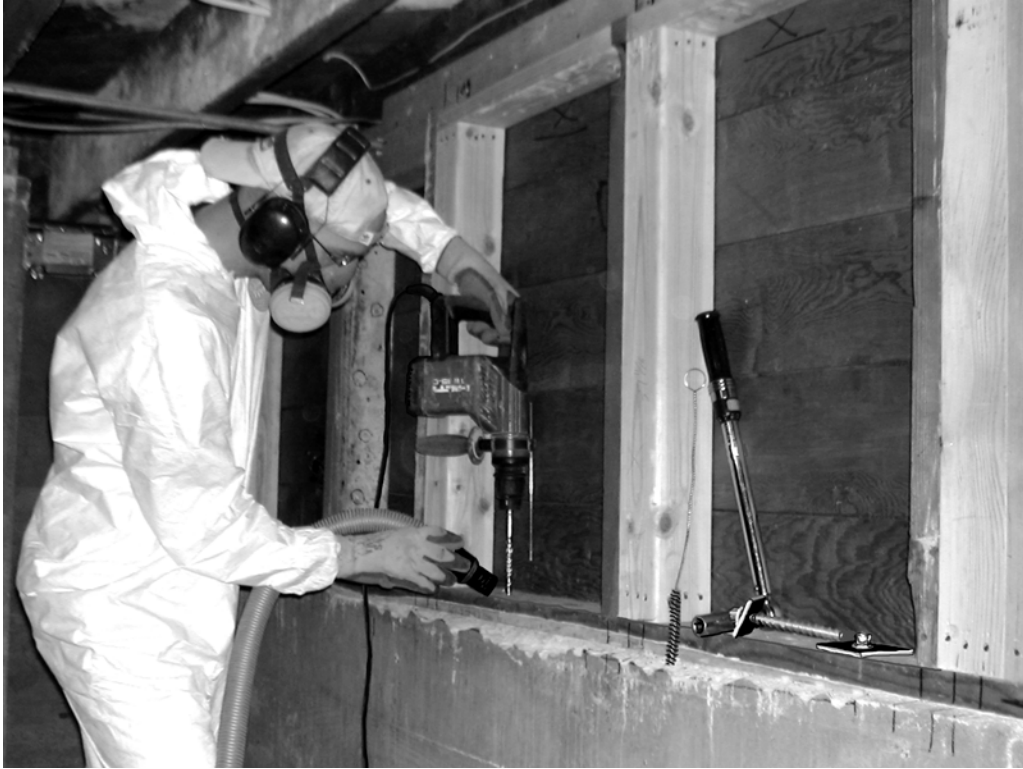
Figure 4 Installing anchor bolts through the sill plate and into the foundation, using a rotohammer. (Photo from Tom Hall)
