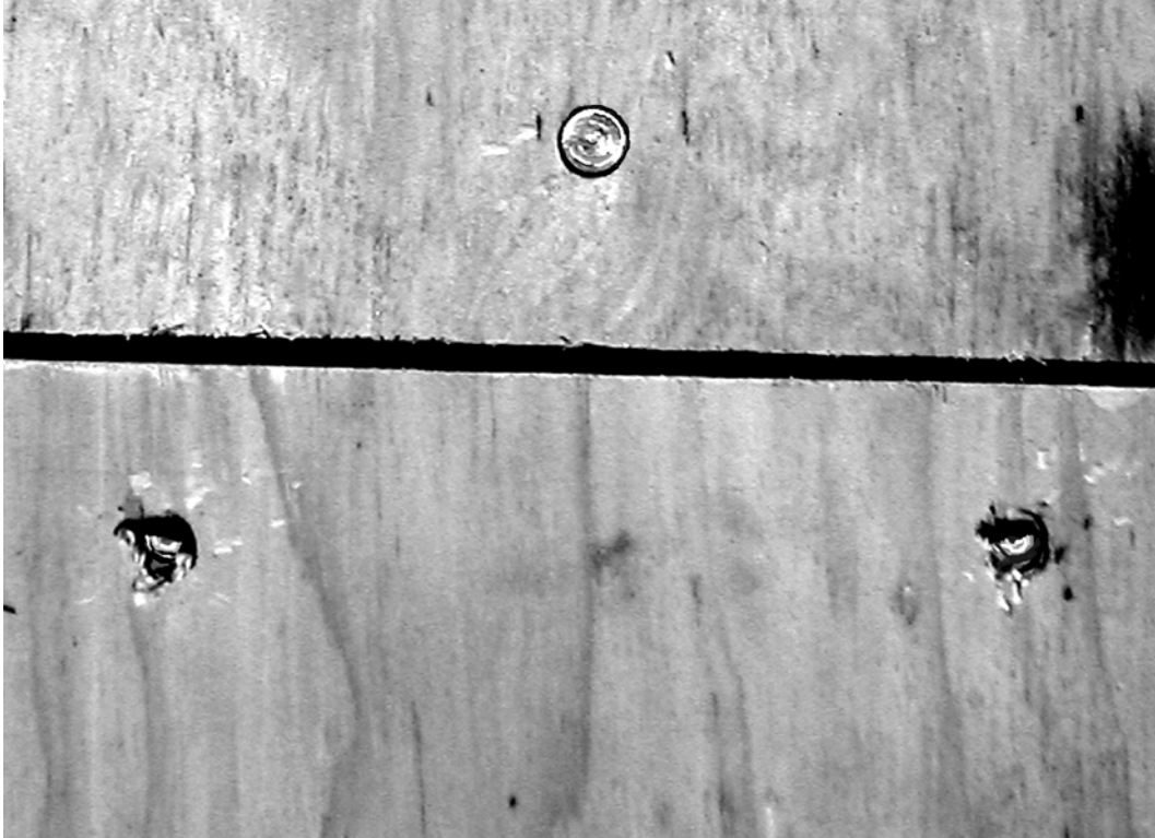
Figure 12 An example of overdriven nails. Nails should be driven flush to the surface of the structural panel, like the top one, and need to be a minimum ½” from the panel edge. (Photo from Tom Hall)
