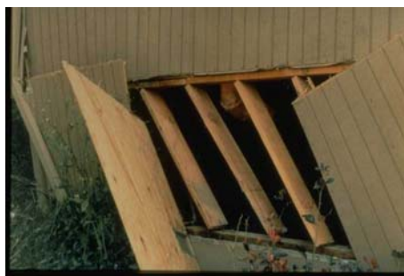
Figure 8 Pony wall failure after the 1994 Northridge Earthquake from excessive side sway. (Photo from FEMA)
