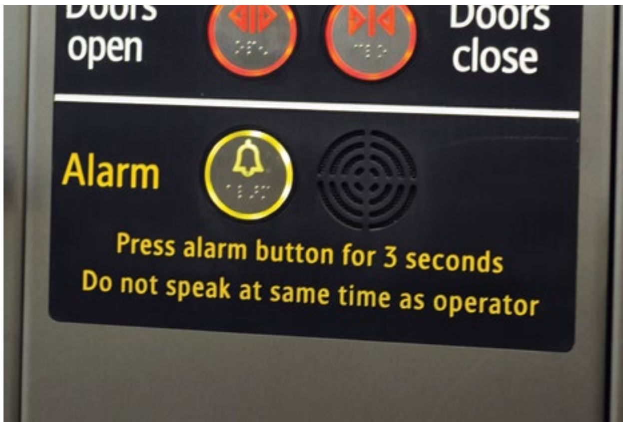
Figure O2.1 Lift controls, showing the alarm button
