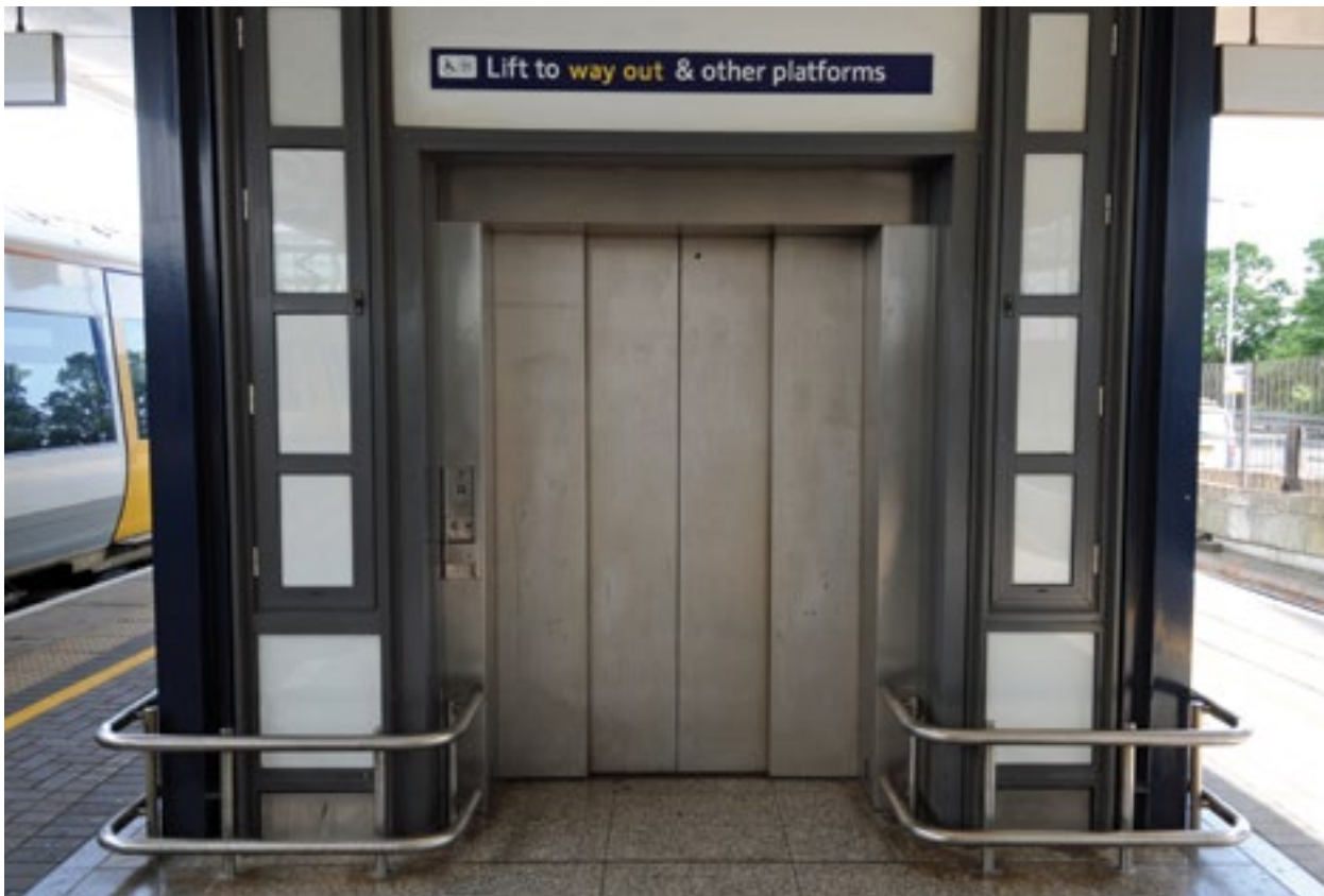
Figure R1.1 A typical station lift
