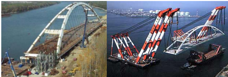
Figure 44 – Arch construction on the riverside, and floating cranes erecting the steelwork – Pentele Bridge (2006) .
