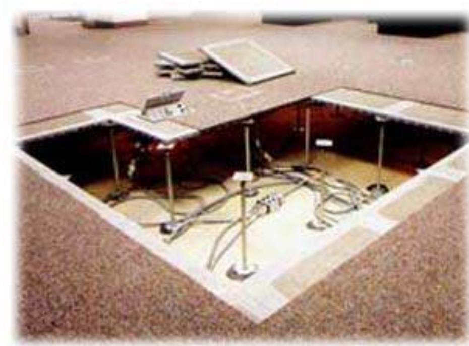
Figure 2-7 : Typical Raised Floor
