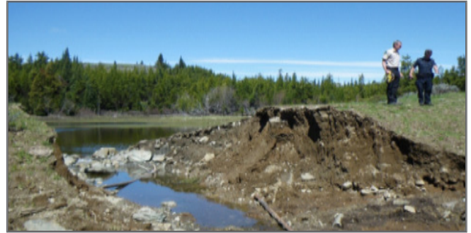
📍 TESTALINDEN DAM Failure (near Oliver) June 13 2010. In 2010, a torrent of mud and debris caused widespread destruction near Oliver after the earthfill Testalinden Dam on an irrigation reservoir failed after heavy rains. A review found that the owner had ignored warnings about the dam's condition.
