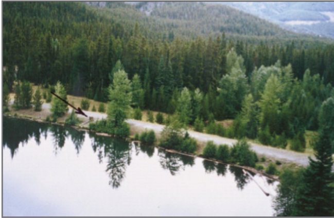
FIGURE 14: Shows a poorly maintained dam with excess vegetation on the slope and a broken log boom
