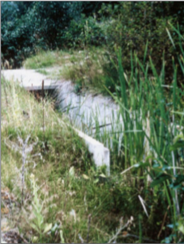
FIGURE 10: Obstructed spillway channel
