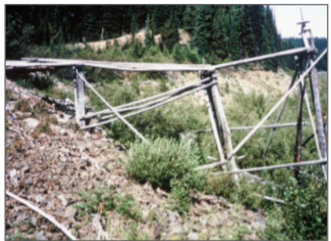
FIGURE 16: Intake control access structure failure
