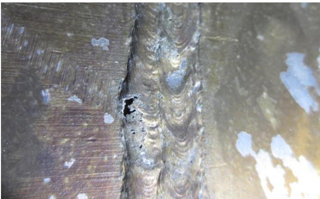
Fig. 3 CORRODED 2205 WELD DUE TO UNDER-ALLOYED WELD METAL
