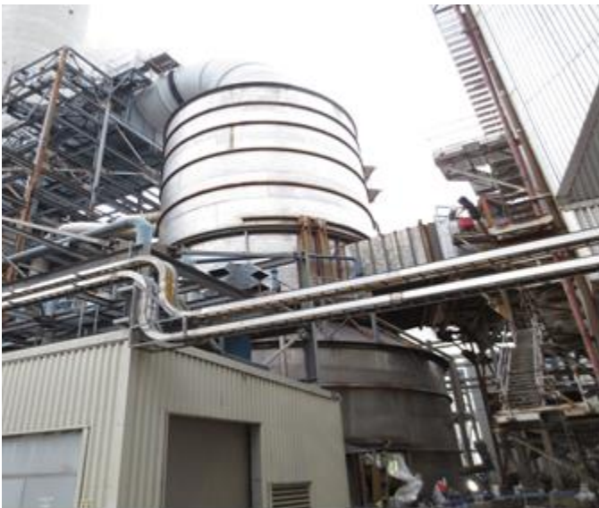
FIG. 1 ALLOY 2205 DSS ABSORBER TOWER AT COAL FIRED POWER PLANT
