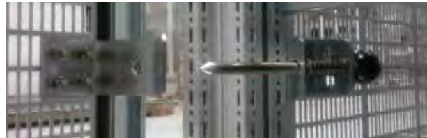
Mechanical door interlock (slam latch) viewed from inside enclosure, not engaged
