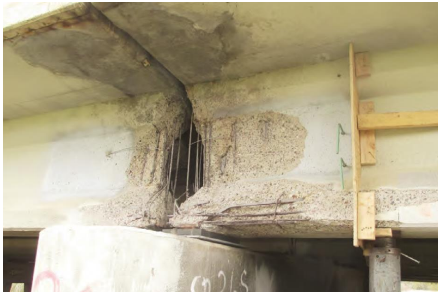
Figure 1.1. Severely corroded prestressed concrete girder (Minnesota)
