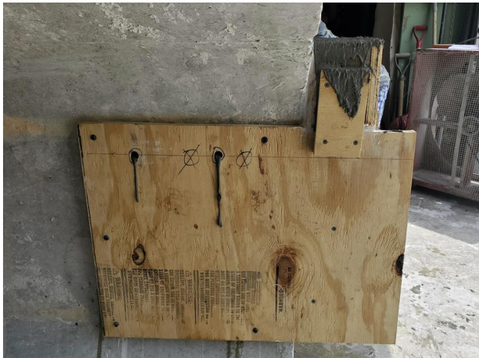
Figure 4.9. Patch mix flowing from weep holes
