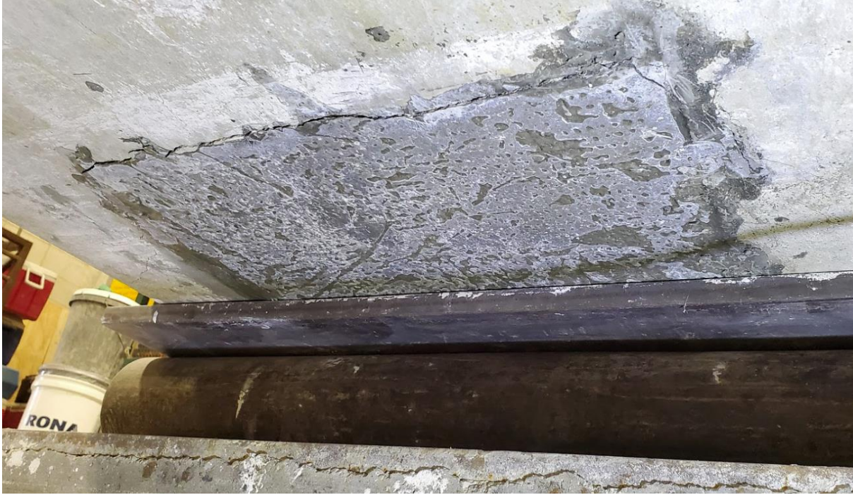
Figure 4.18. UHPC-2 south flange patch cracking along interface
