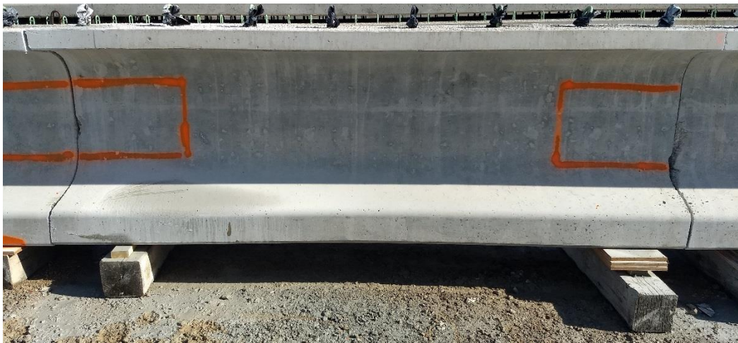
Figure 4.3. Cut beam segment marked for artificial damage
