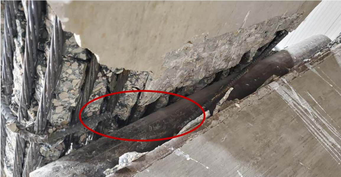
Figure 4.14. Fractured stirrup on bottom flange of Control-2
