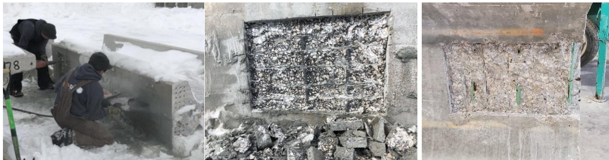
Figure 4.5. Cutting and chiseling (left), damaged bottom flange (center), and damaged web (right)
