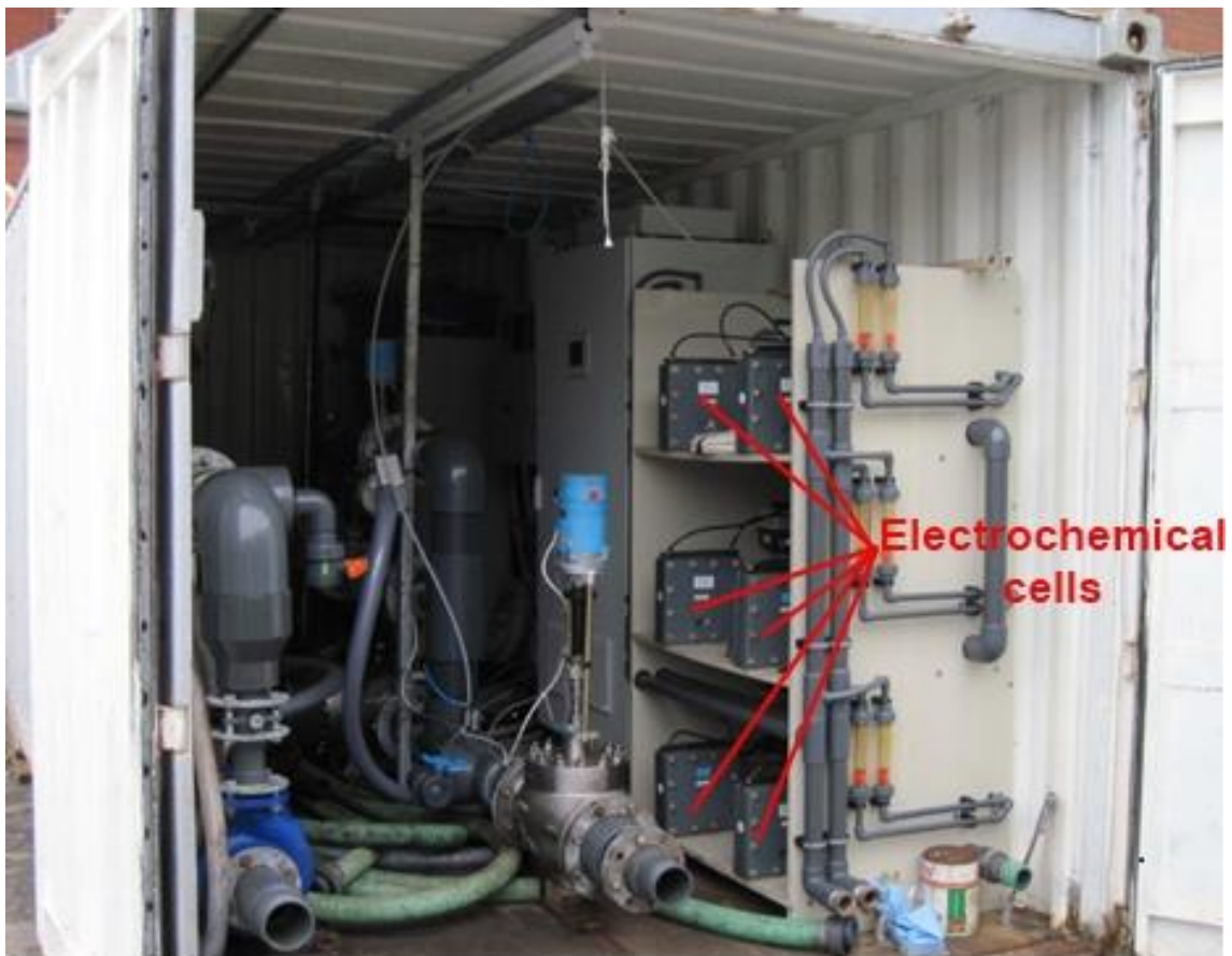
Figure 10. BaWaPla Pilot System, Blyth-England (2009).
