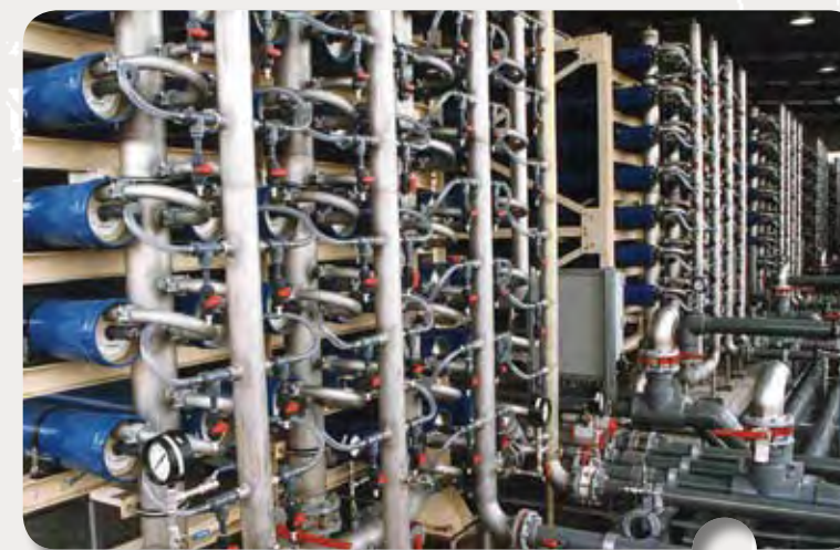
30,000 M 3 /Day Reverse Osmosis Installation
