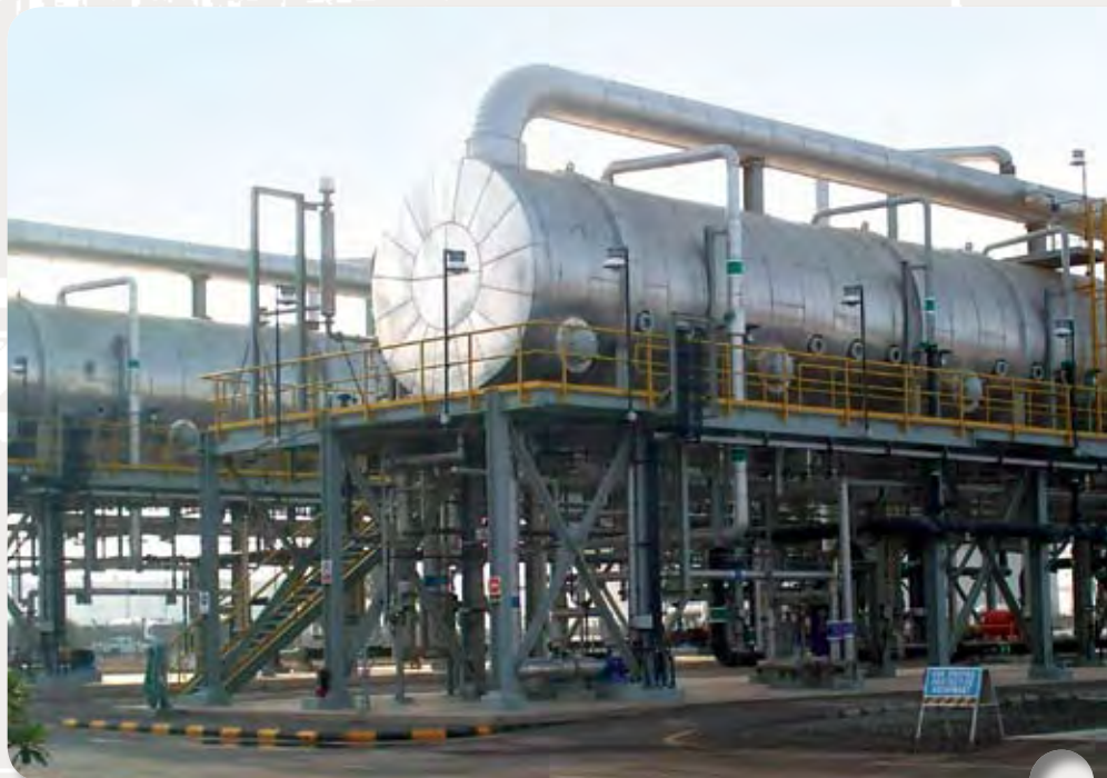
This 10,000 M 3 /Day MED Plant, at Aramco's Rabigh Refinery, is Saudi Arabia's first industrial BOOT project.
