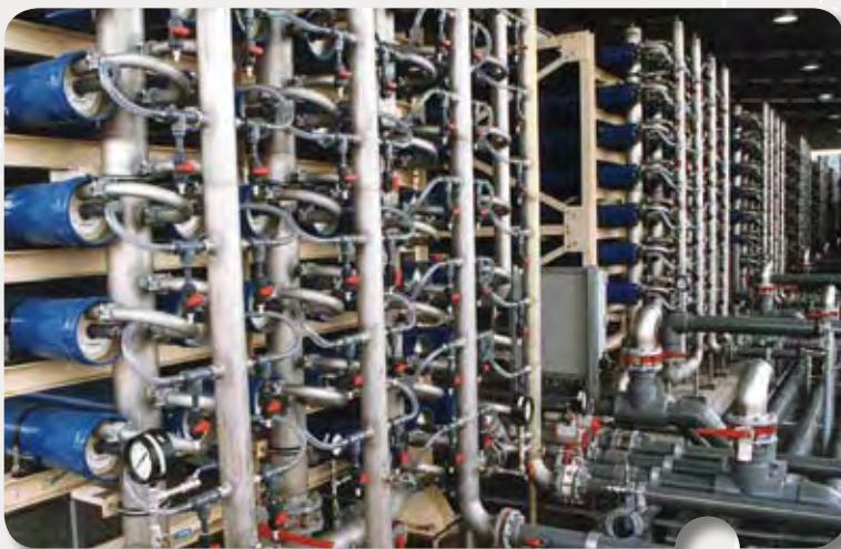
30,000 M 3 /Day Reverse Osmosis Installation
