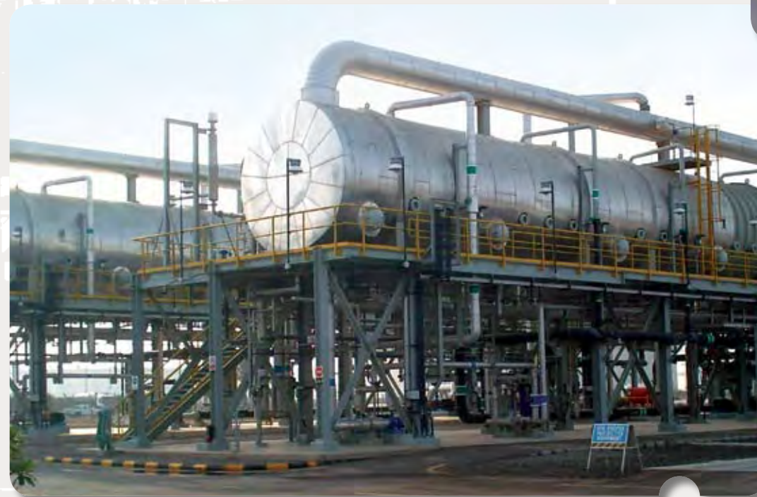
This 10,000 M 3 /Day MED Plant, at Aramco's Rabigh Refinery, is Saudi Arabia's first industrial BOOT project.
