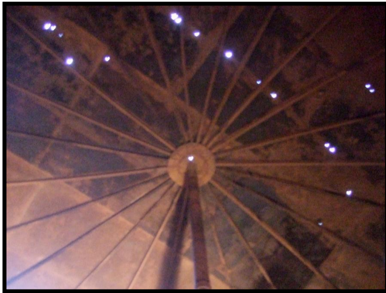
Severe roof corrosion
