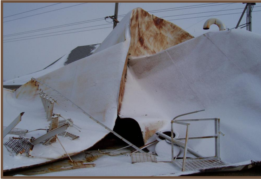
Double wall 500,000 gallon tank, Illinois 2008
