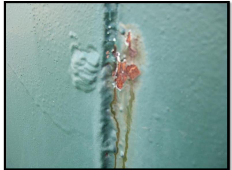
Lap-welded seam leak
