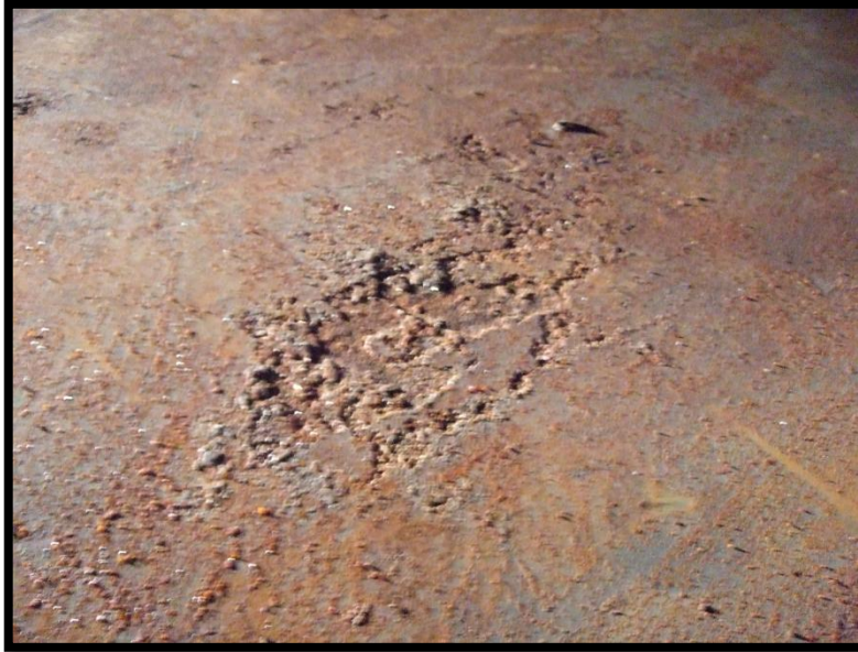
Floor plate corrosion
