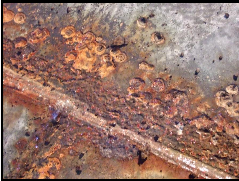
Floor top side corrosion
