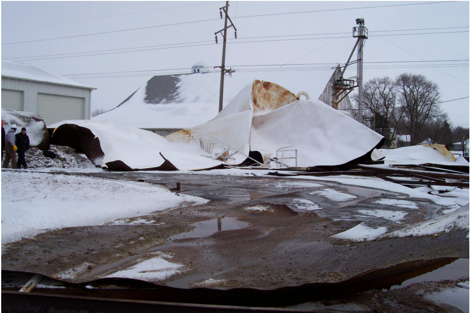
Weld seam rupture. Force of rupture “pushes back”. Rupture on side of camera location.
