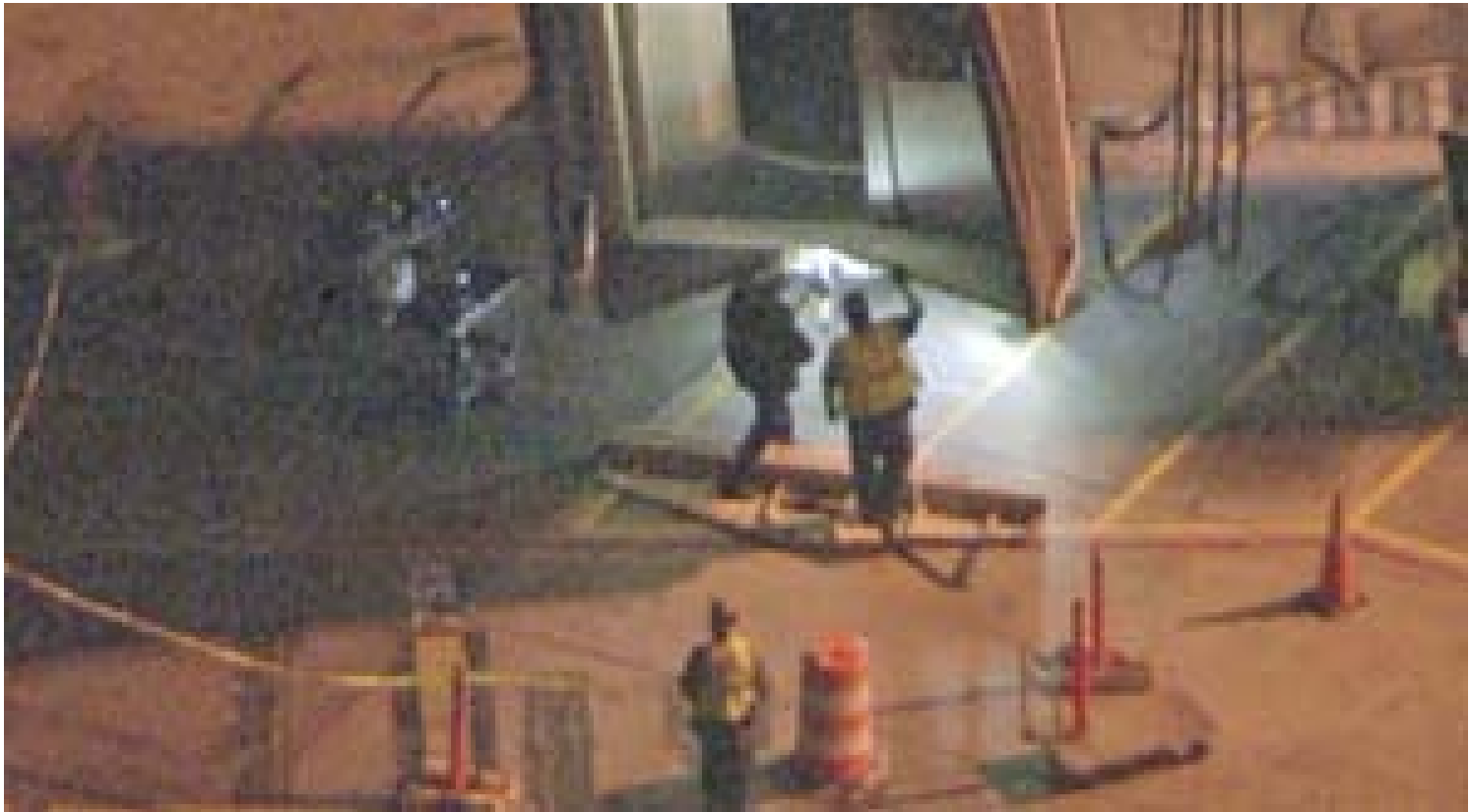
Photo: Crews inspect jet bridge damage. Credit: KTLA-TV News LA Times
