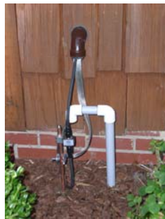
Shack end - Ground Rod and PolyPhaser protection
