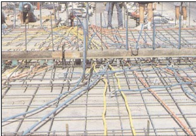
Carlson ENT roughed-in a deck (between layers of rebar) ready for a concrete pour (tunnel form).
