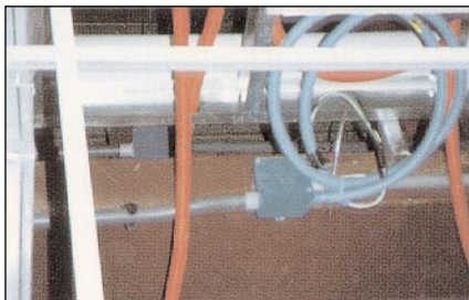
ENT above a suspended ceiling (ENT fixture whips)
