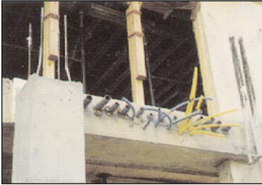
ENT in a Floor Slab prepared for more form work to extend conduits in the next pour.
