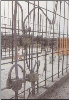
ENT terminated on a Switch Box ready for a poured concrete wall. (This is a Tunnel Form Method).
