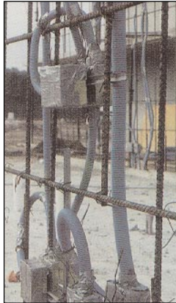
Tunnel Forming project Carlson ENT terminated in metal* boxes roughed-in for a poured concrete wall
